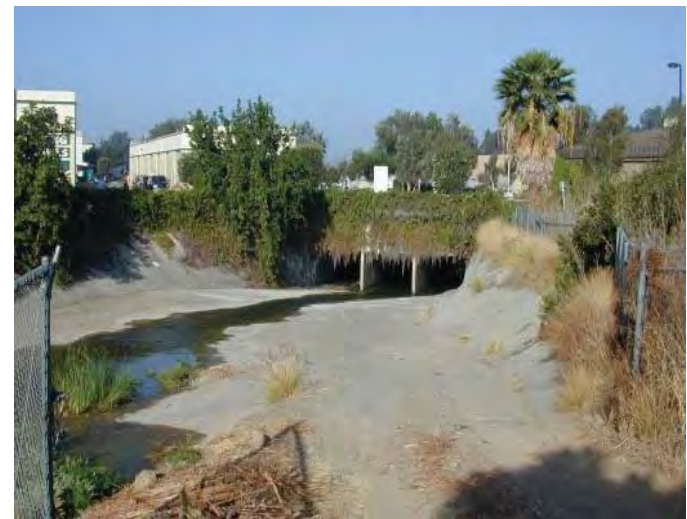
The channelization of Alvarado Creek above the Grantville Post Office offers little wildlife habitat and allows for no groundwater recharge
