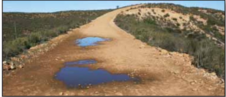
Utility road maintenance grading has created berms along the edges preventing proper drainage
