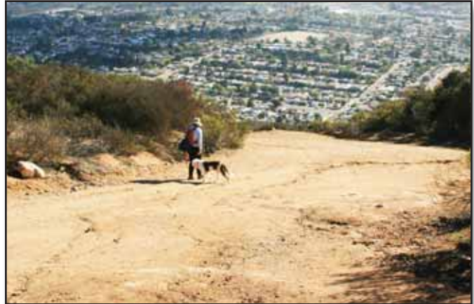
Eroding drainage swales along section of Cowles Mountain service road (CM-M1)
