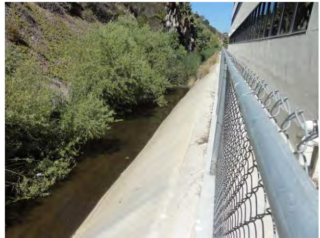
From North side of channel, at start of Reach 3, where channel becomes 100% concrete, looking downstream
