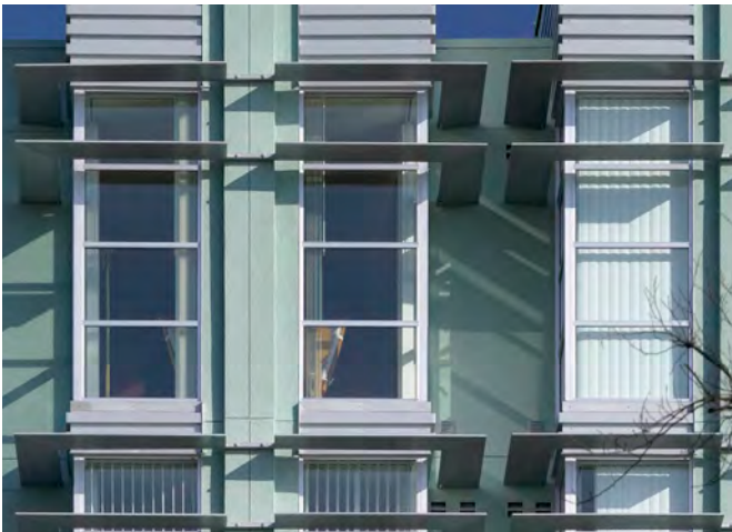
Sunshades may be included on upper stories or lower stories to shield solar rays into building interiors.
