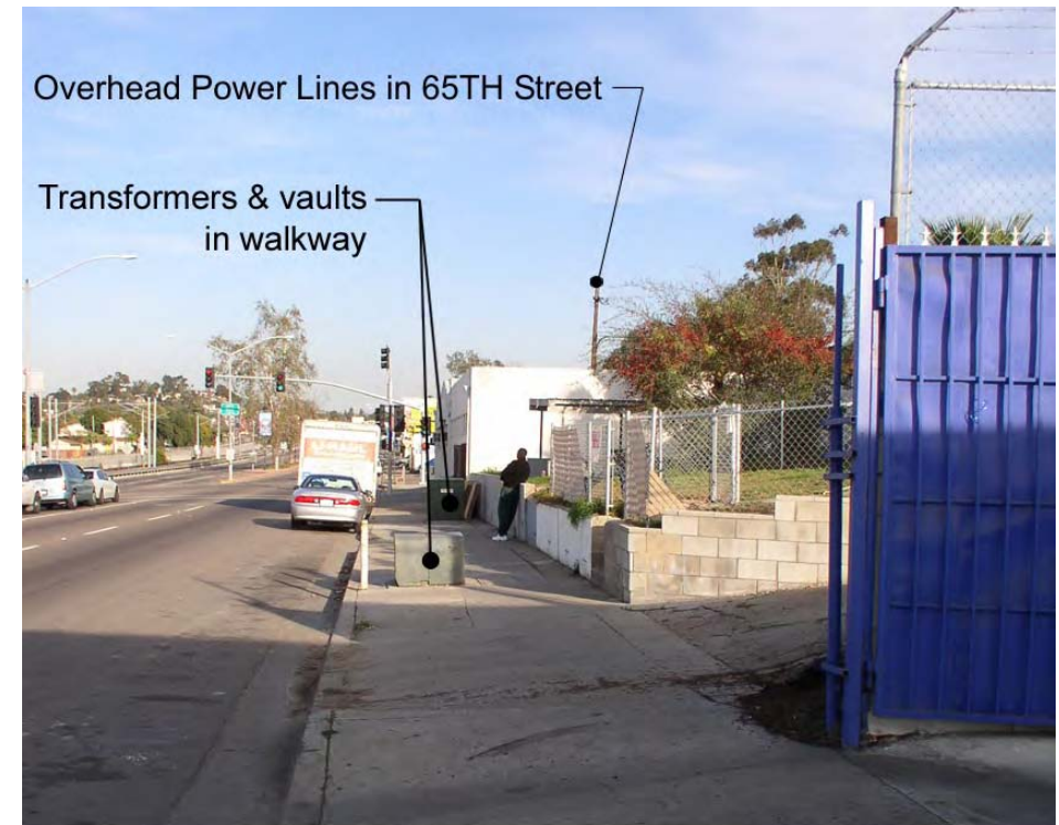
Exhibit 6.10 Existing Transformers and Vault
