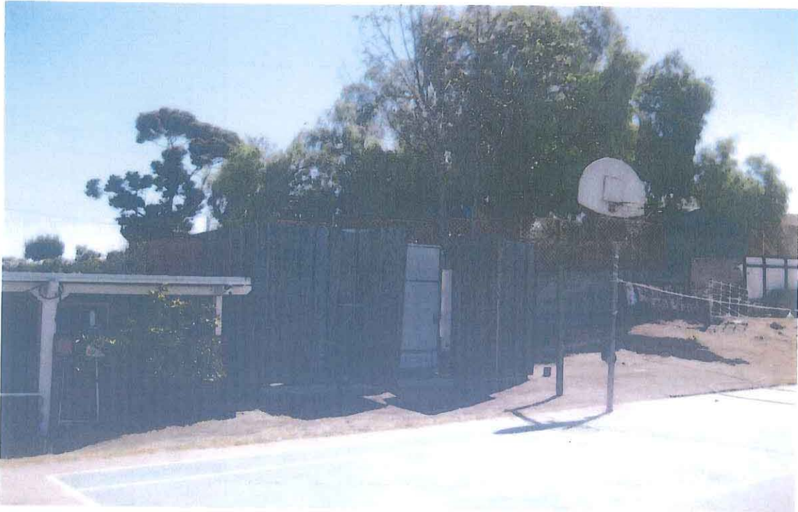
Existing AT&T Equipment Enclosure and Equipment
