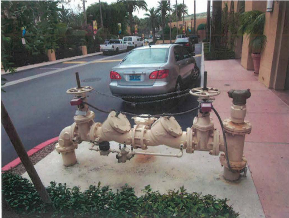
35) View of double check valve assembly for the fire water system.
