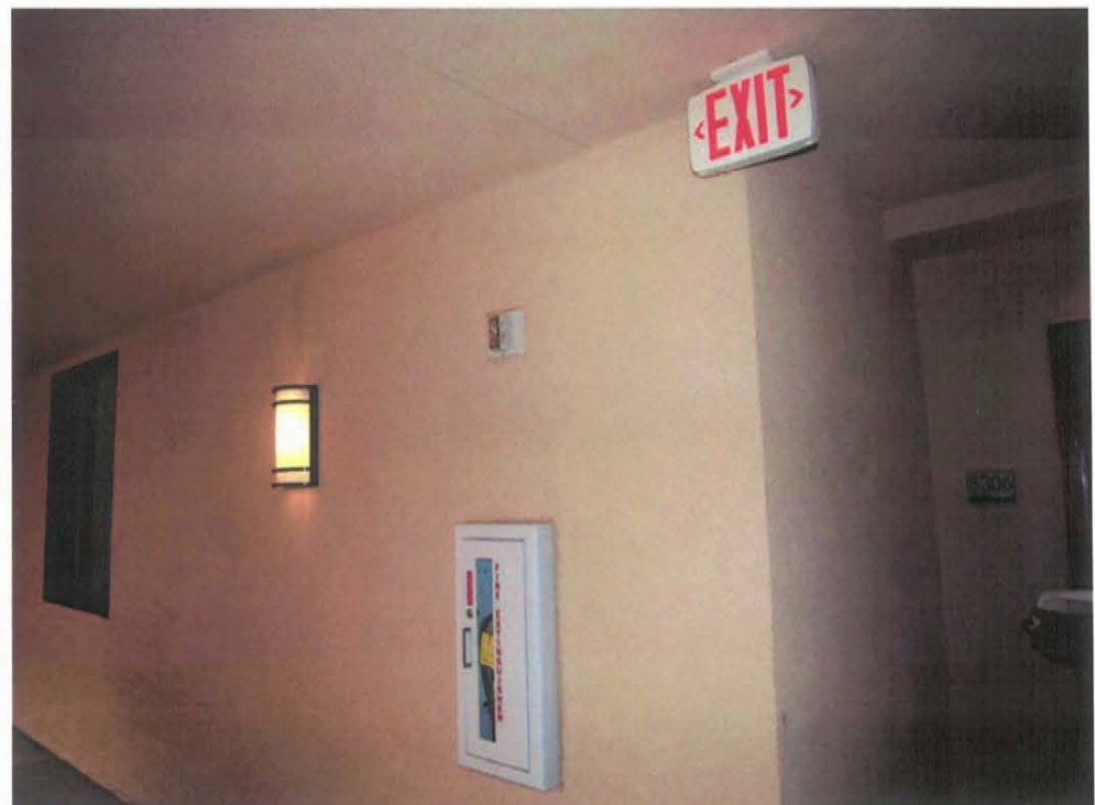
34) Typical of lighted exit signage, fire extinguishers and audible/visual alarms with strobe light.
