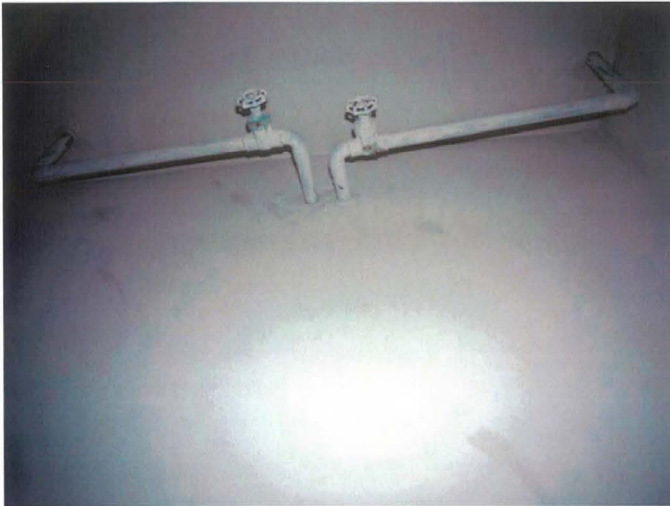
33) Typical piping to be used for future individual water meter connections in unit closets.
