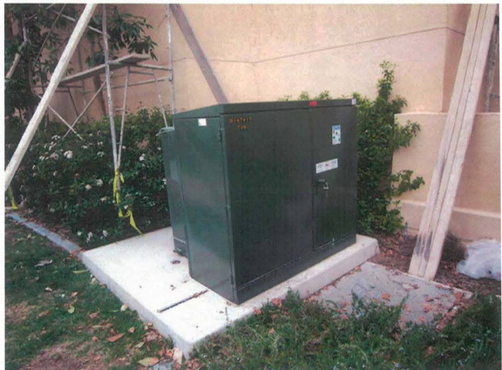
36) Typical of main electrical transformers on site.
