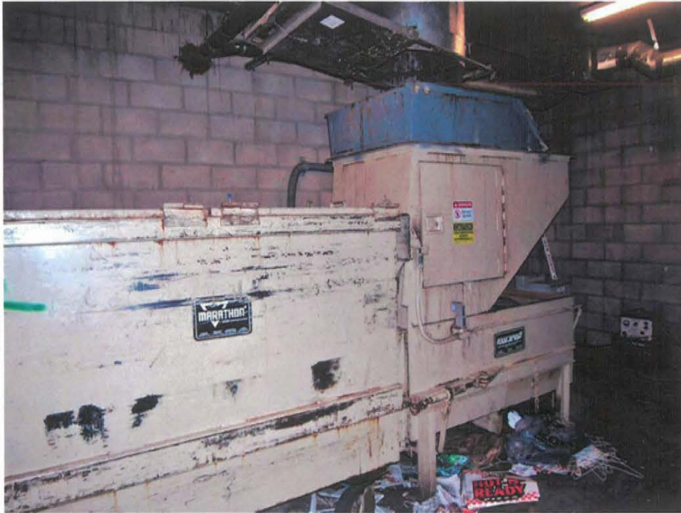
37) View of trash compactor and bin located beneath garbage chute
