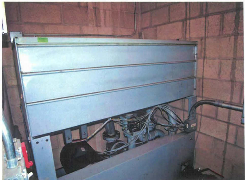
38) Typical of elevator equipment.
