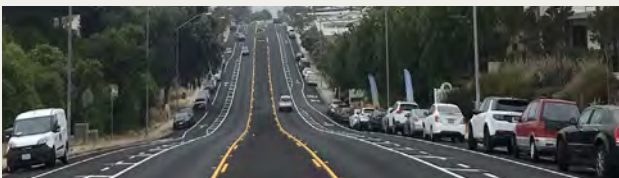
Road resurfacing with bikeway on Gramercy Drive Source: City of San Diego
