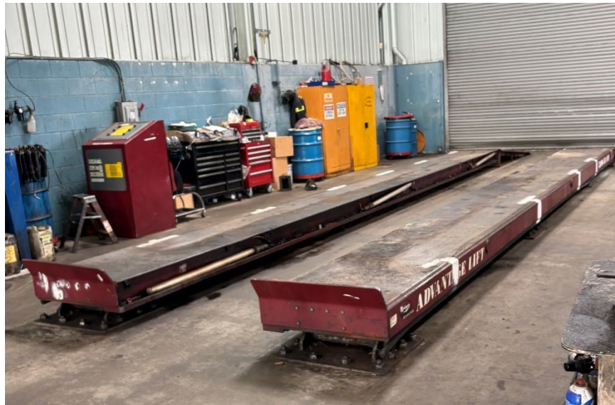
Figure 8-2 Platform Lift for Preventative Maintenance of Vehicles
