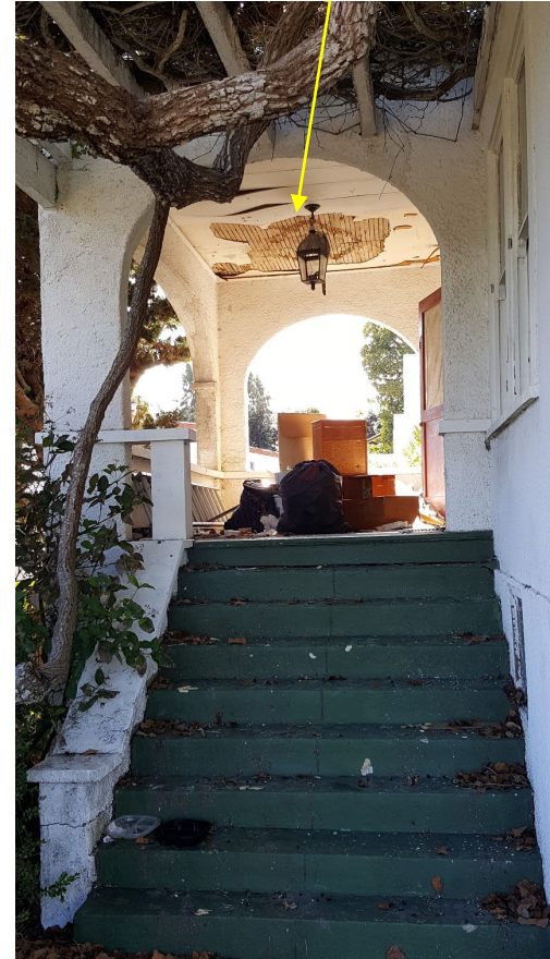
Porch Detail—Note Deteriorated Porch Roof Condition
