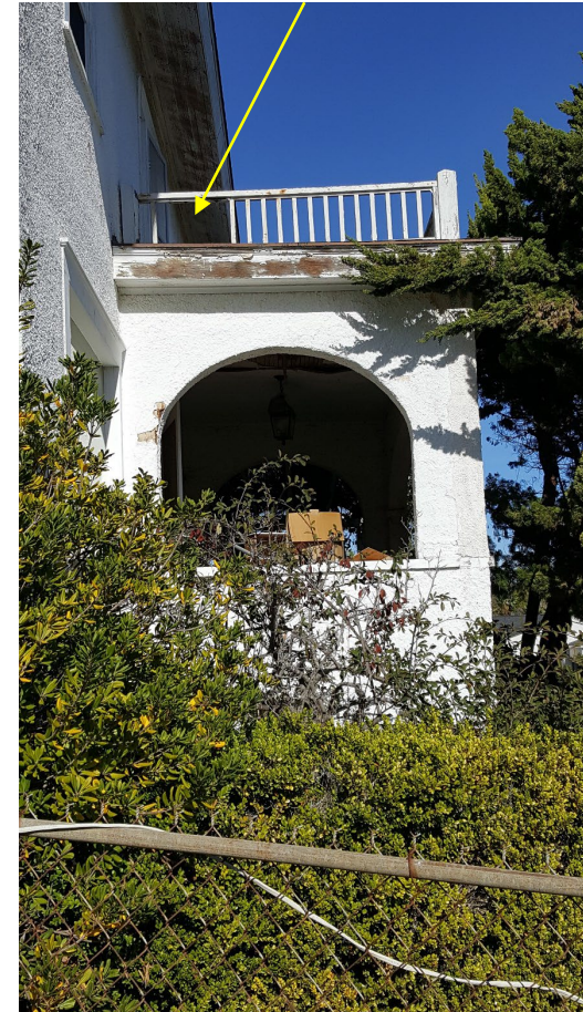
Note Missing Balusters
