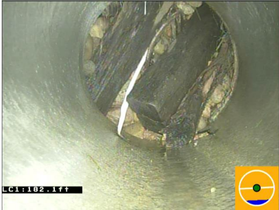
CCTV looking upstream of plugged 30-Inch RCP
