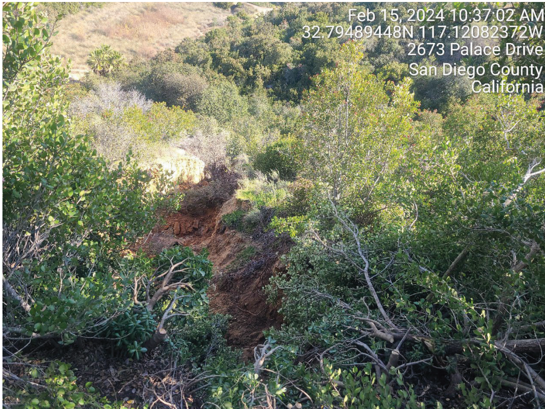
View of sinkhole from Upstream
