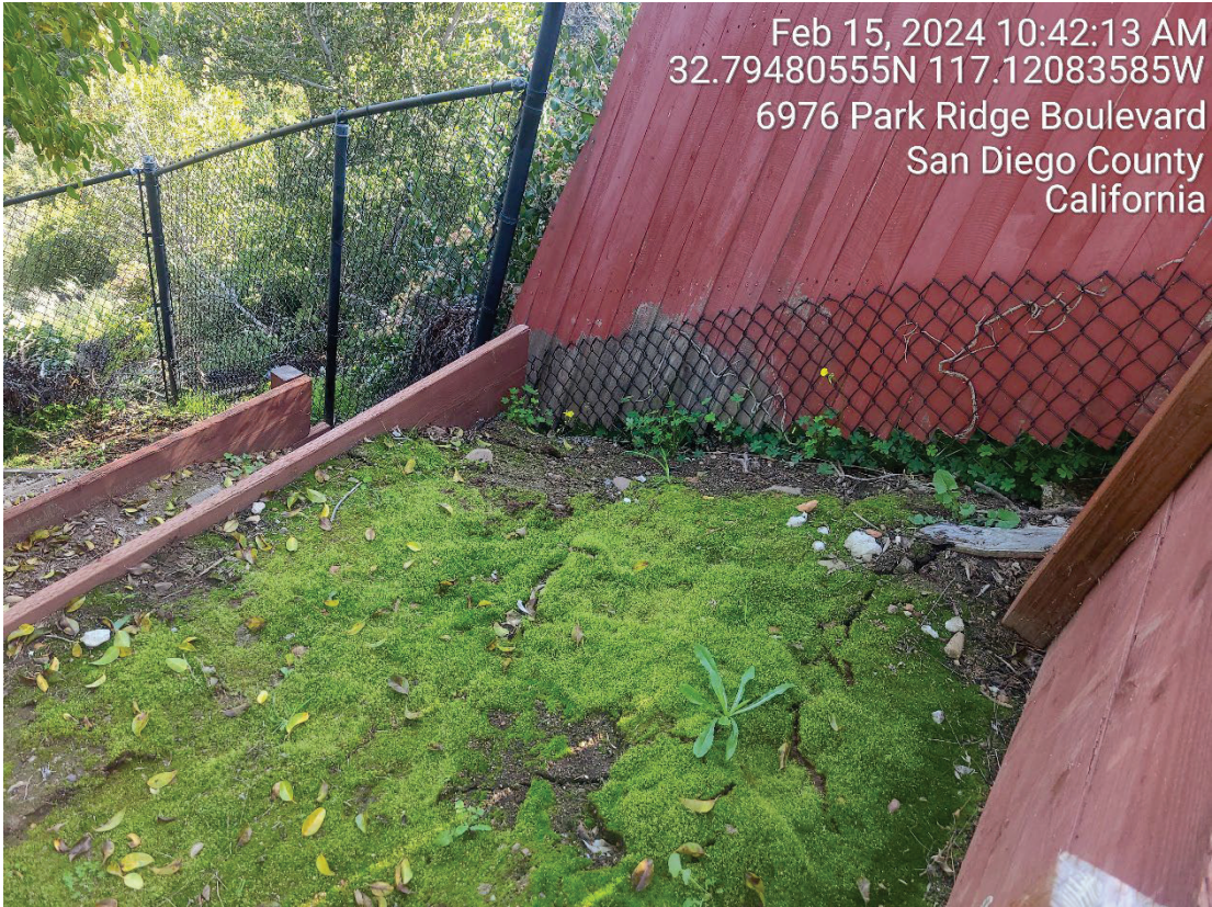
Fissures and cracking of slope within 2681 Palace Drive
