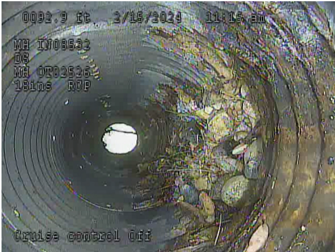
Corroded 18-inch CMP from CCTV Survey from February 15, 2024
