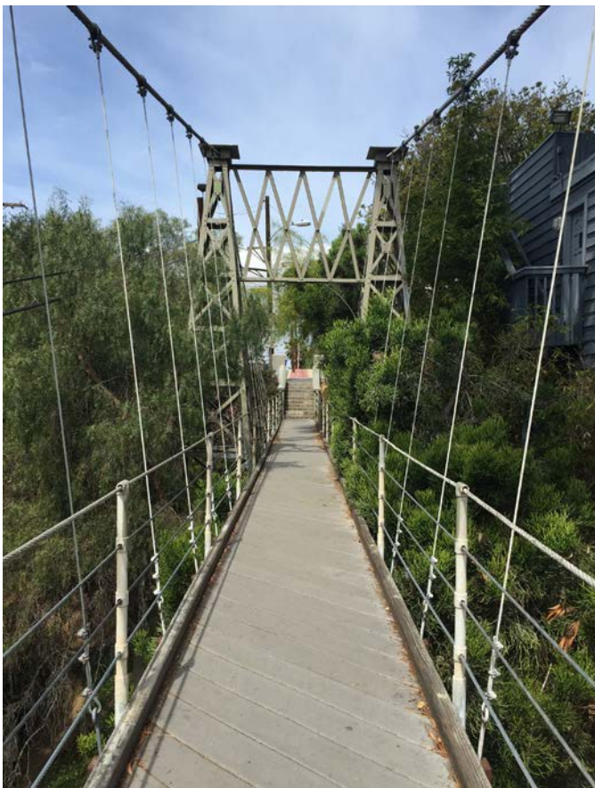
The Spruce Street Bridge, engineered by Edwin Capps, still provides access over Arroyo Canyon since its completion in 1912.
