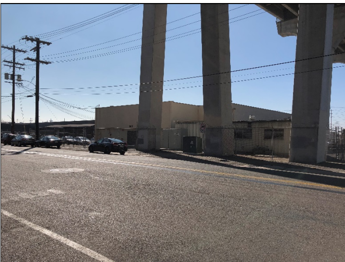
35. View of southwest-adjacent pad-mounted transformer
