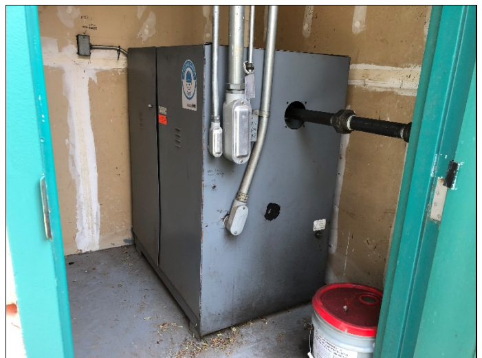
6. View of elevator equipment room
