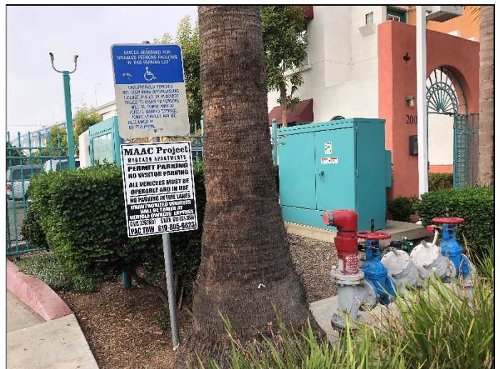
12. Representative view of pad-mounted transformer located on the subject property
