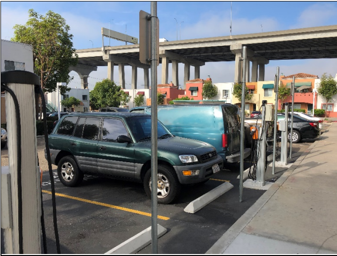
13. View of the electric vehicle charging stations
