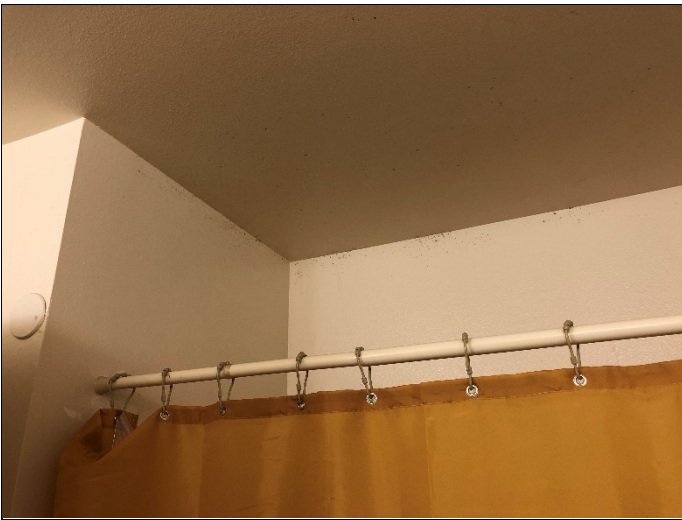
21. Representative view of mold growth observed in bathroom units
