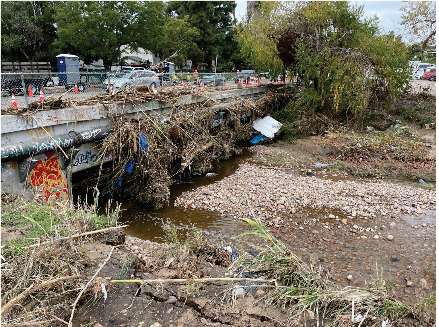
47 th St and Castana St – Looking west at channel. Sediment, debris, and vegetation blocking pathway under bridge. The blockage will need to be cleared before next rain event.
