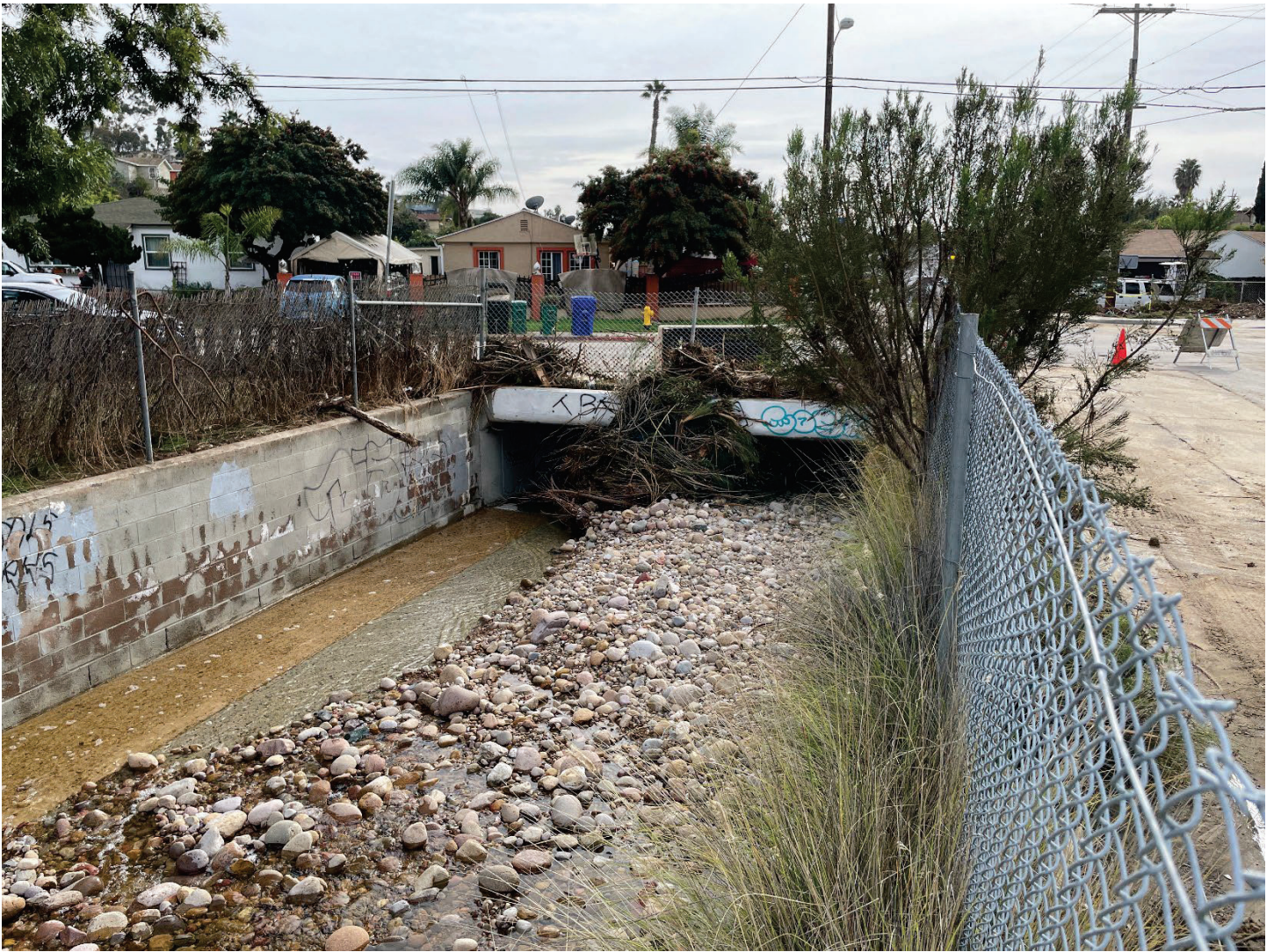
Intersection of Elwood Ave and Geneva Ave – Looking south at channel. Sediment, debris, and vegetation blocking pathway under bridge. The blockage will need to be cleared before next rain event.
