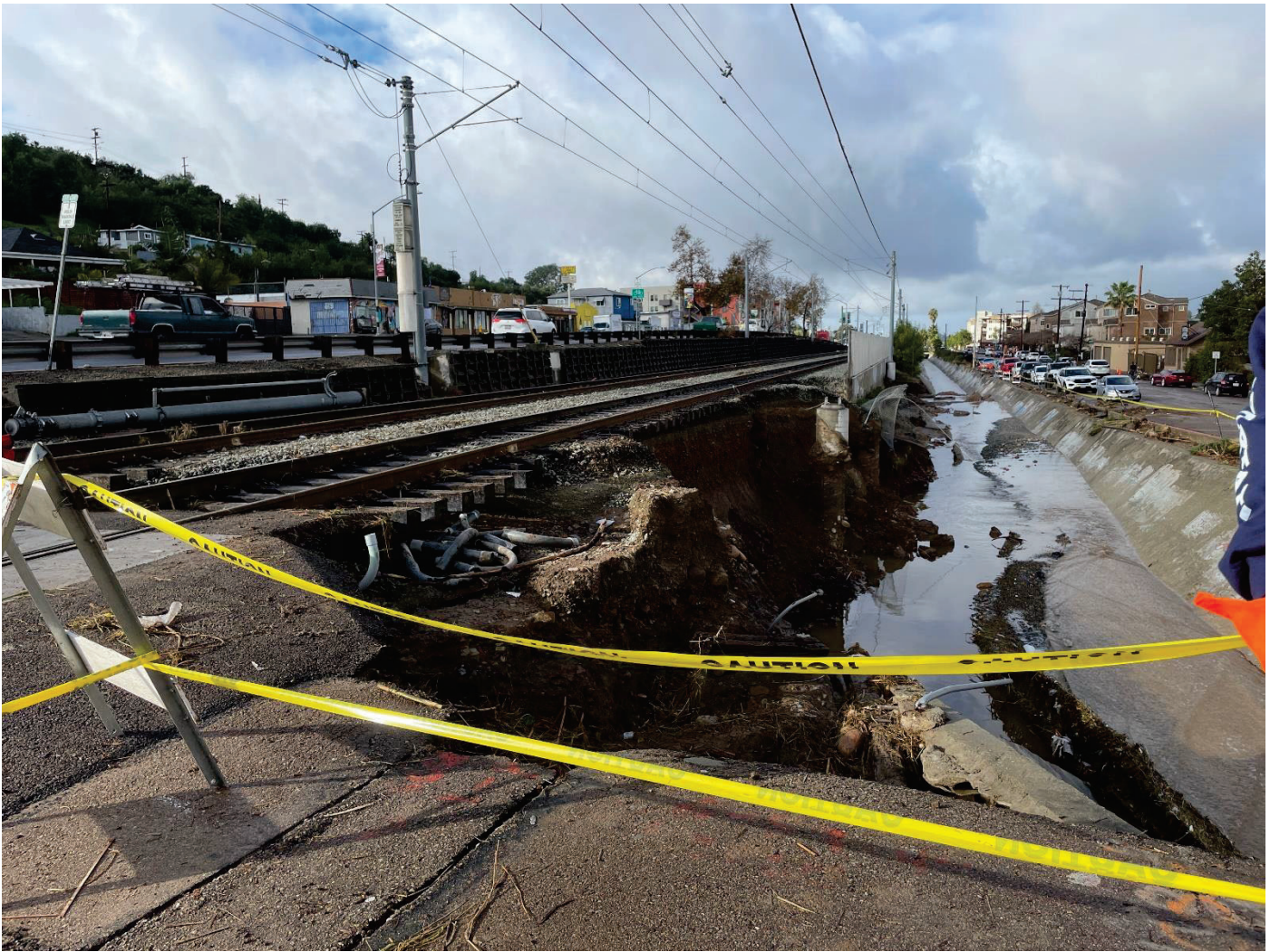
6474 Akins Ave – Looking southwest at MTS trolley tracks and Imperial Ave. Water breaching channel and onto MTS trolley tracks causing damage to the trolley tracks, trolley wires, and trolley retaining wall. Concrete channel is also damaged.
