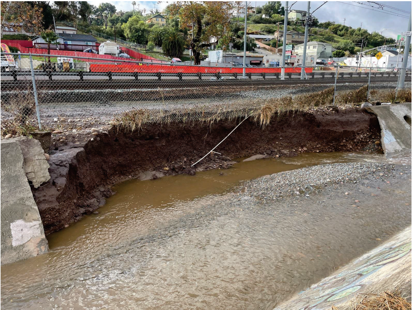
6540 Akins Ave – Looking southwest at MTS trolley tracks and Imperial Ave. Water breaching channel and onto MTS trolley right of way causing undermining under the chain link fence. Concrete channel is also damaged.
