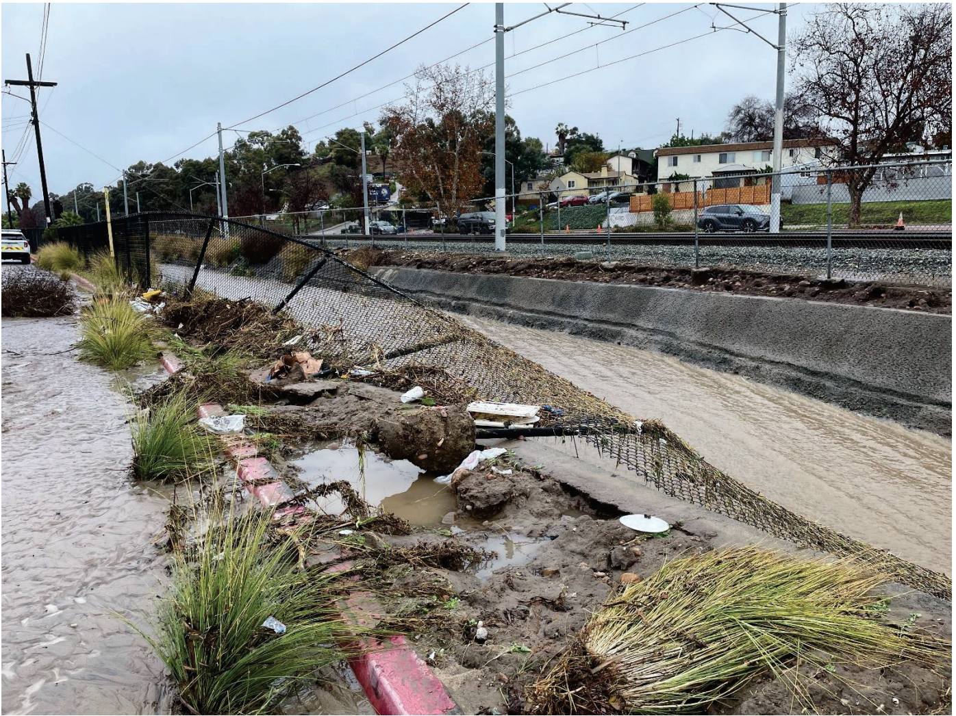
6922 Akins Ave – Looking southeast at channel. Water breaching onto roadway damaging fence, undermining the soil beneath the concrete and flooding adjacent properties
