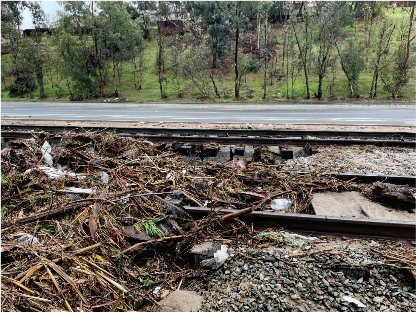
1366 San Altos Pl – Looking south at MTS trolley tracks and Imperial Ave. Water breaching channel and onto MTS trolley tracks causing damage to the tracks.
