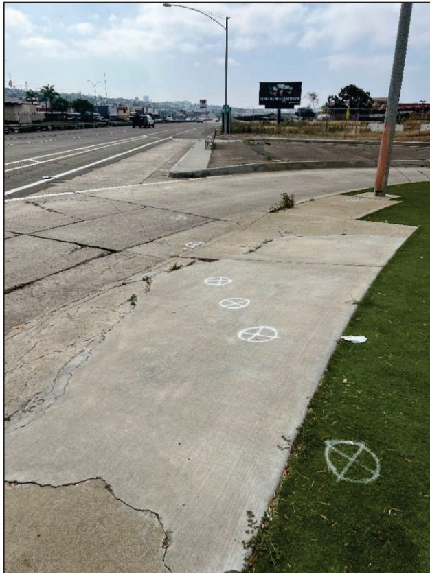
June 12, 2024 – Markings of approximate locations of failures identified during televising on Pacific Highway facing SB
