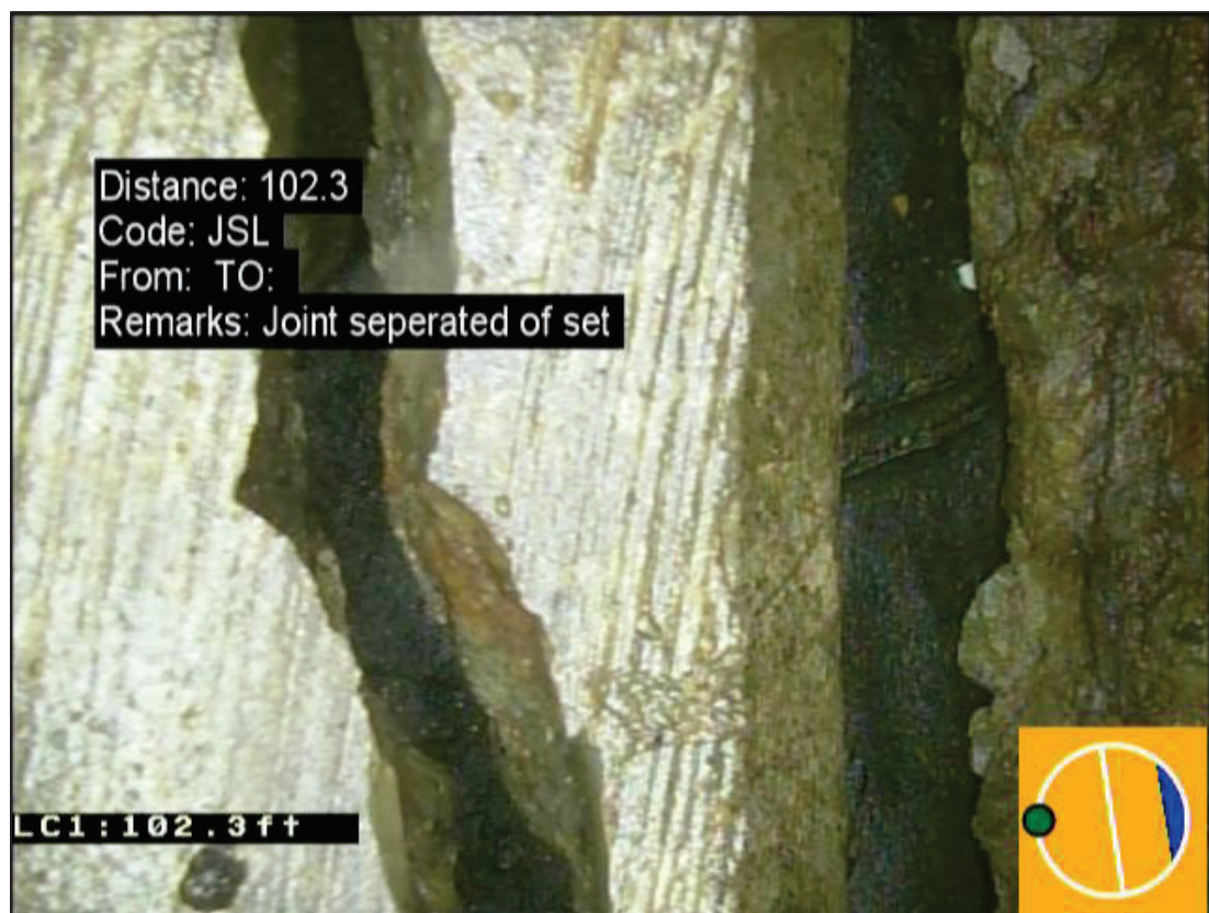
June 13, 2024 – Northern Discharge severe separation of pipe
