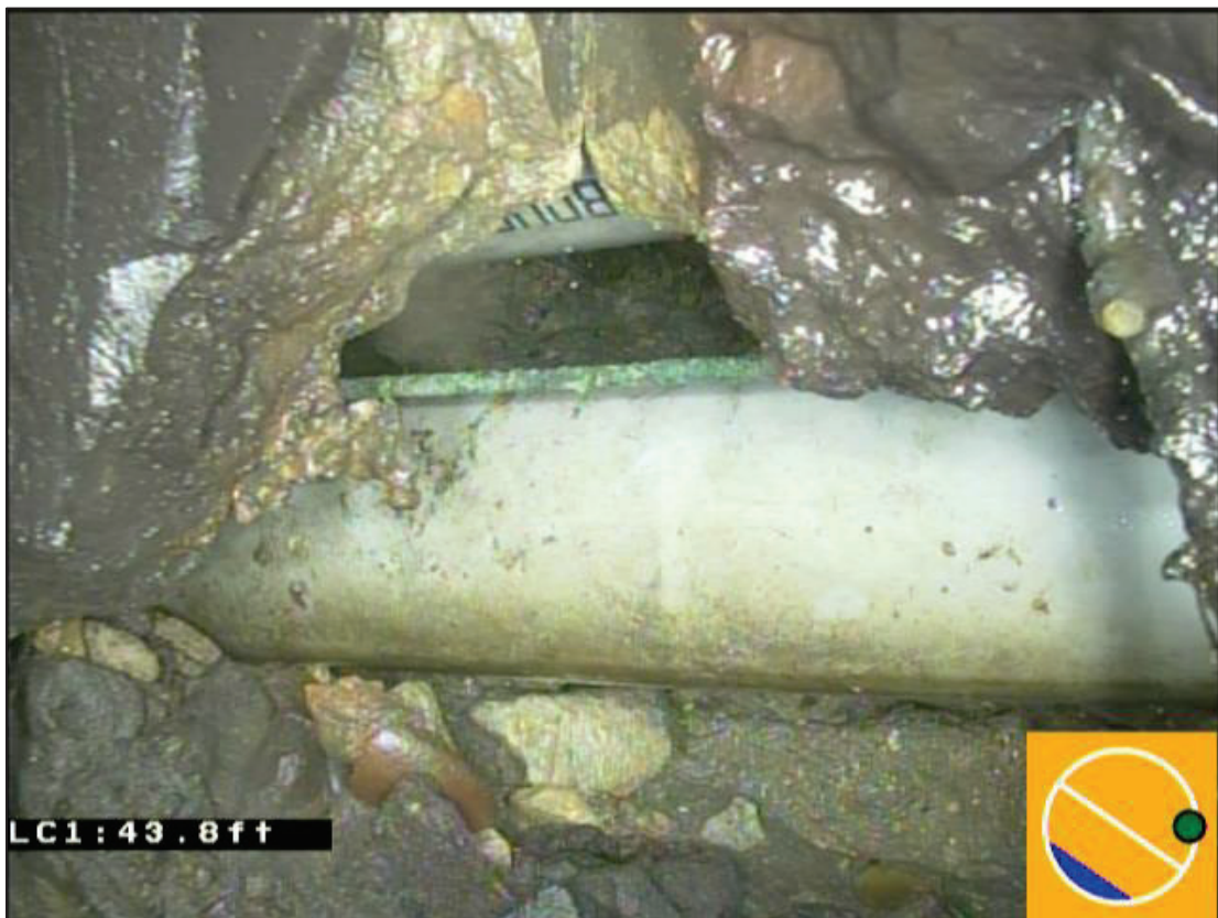
June 12, 2024 – Southern Discharge damage to pipe wall due to conduit trench
