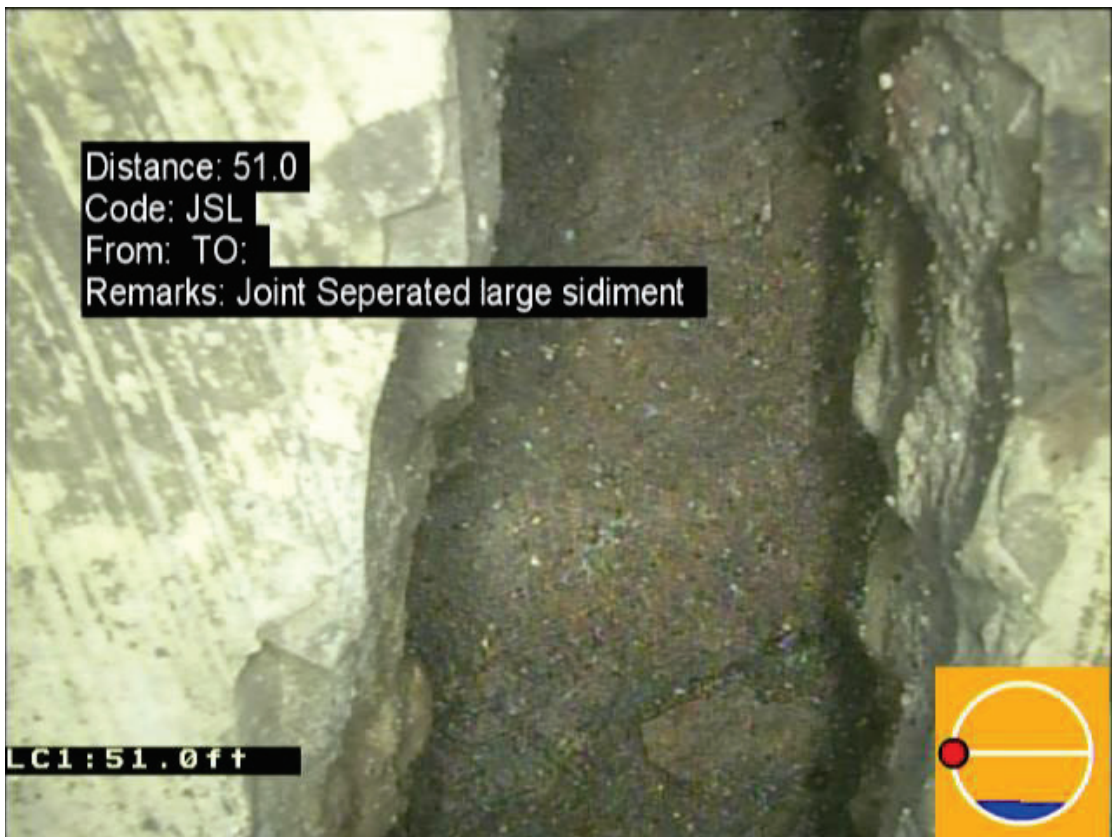
June 13, 2024 – Pacific Highway Crossing severe separation of pipe
