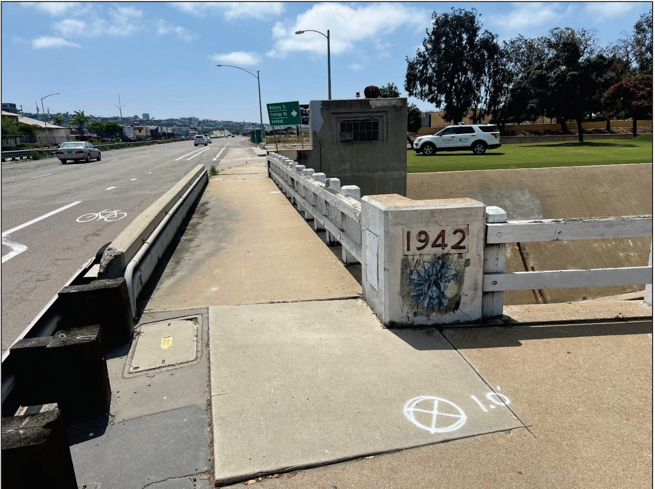
June 13, 2024 – Markings of approximate locations of failures identified during televising on Pacific Highway along discharge north of pump station
