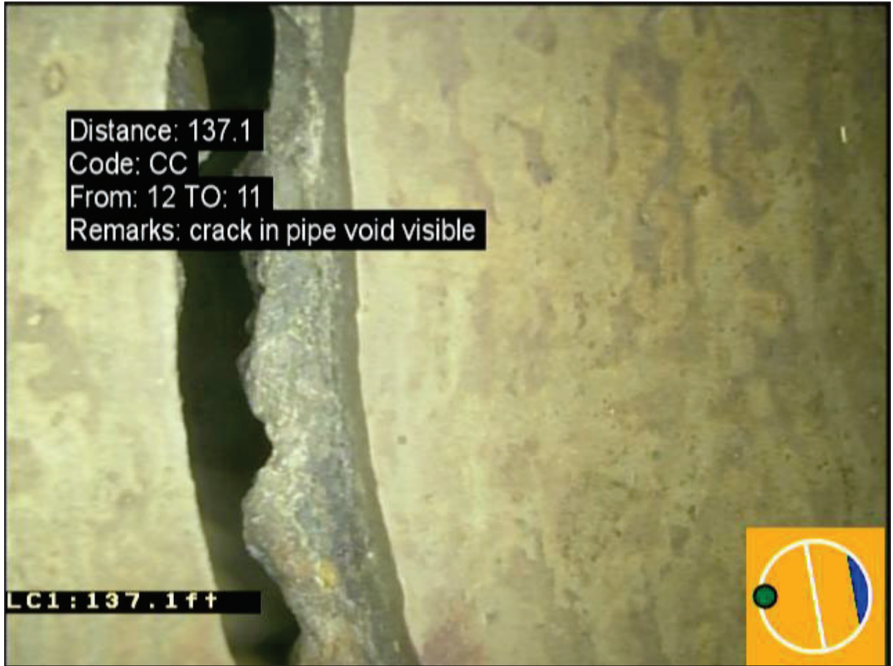
June 12, 2024 – Southern Discharge void observed though crack and pipe separation
