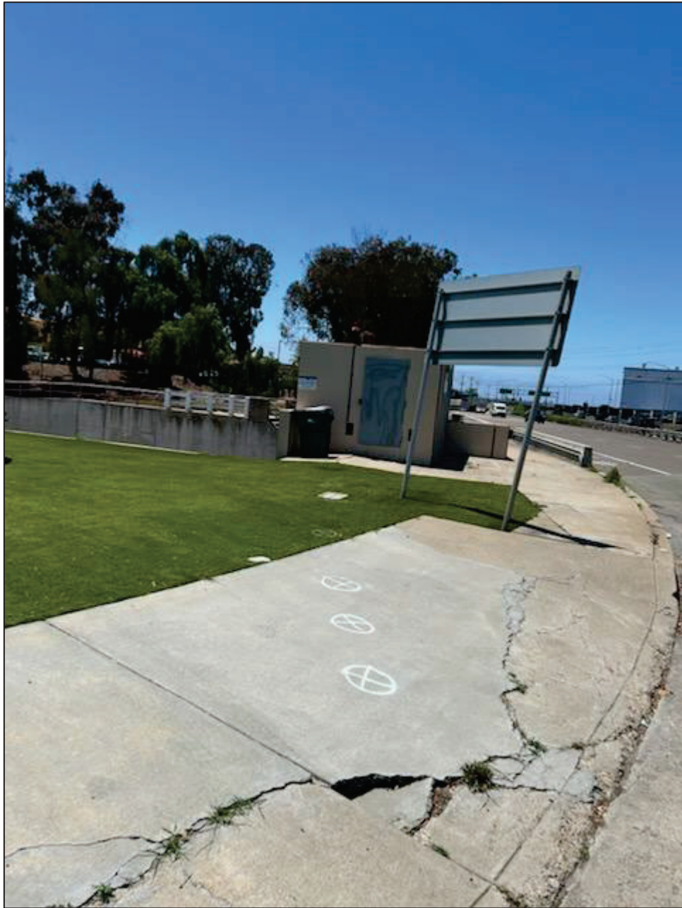
June 12, 2024 – Markings of approximate locations of failures identified during televising on Pacific Highway facing NB.
