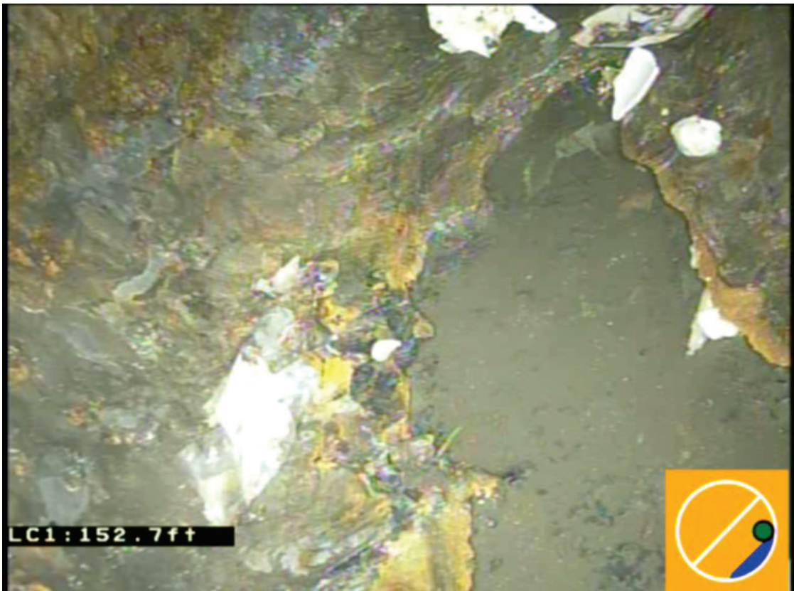
June 13, 2024 – Northern Discharge void developing at bottom of pipe at 90 degree DI turn.
