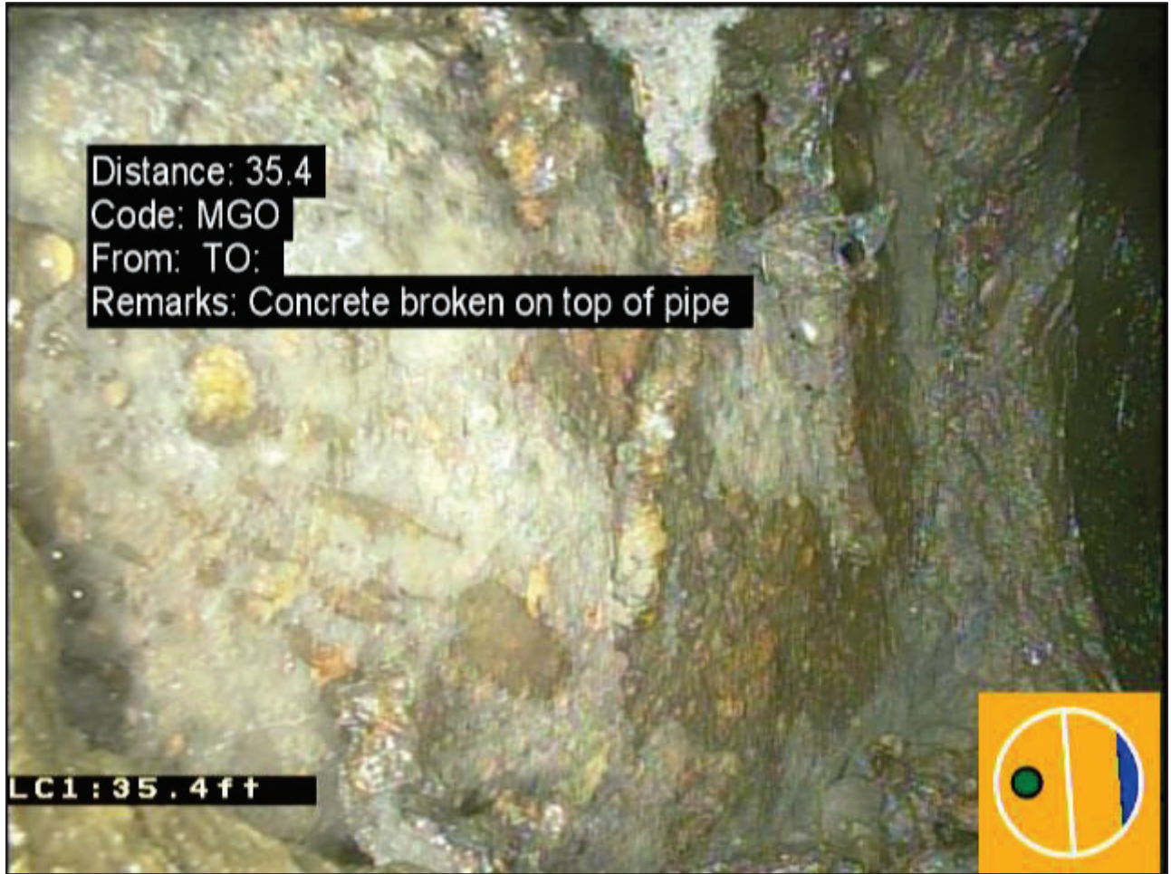
June 12, 2024 – Southern Discharge damaged top of pipe
