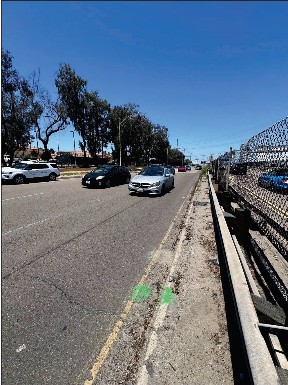
June 1, 2024 – Approximate location of severe cracking in pipe crossing Pacific Hwy
