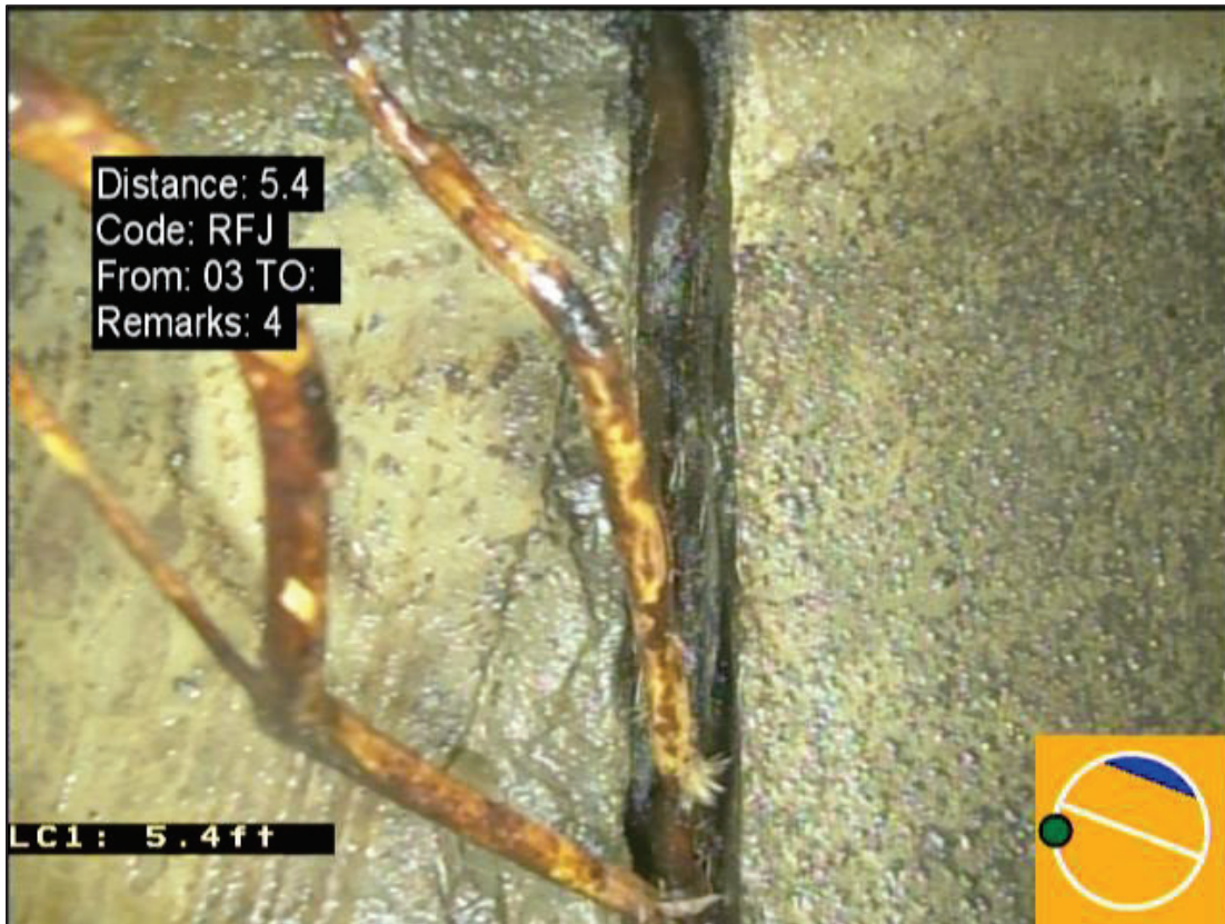
June 13, 2024 – Northern Discharge pipe separation due to tree roots
