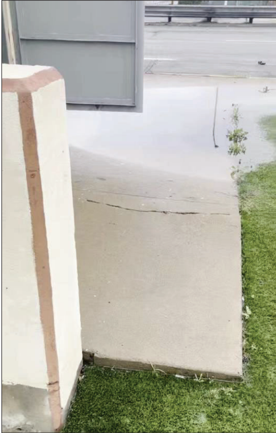
Jan 22, 2024 – Concrete cracking, soil subsidence and water pooling at entrance of Pump Station B
