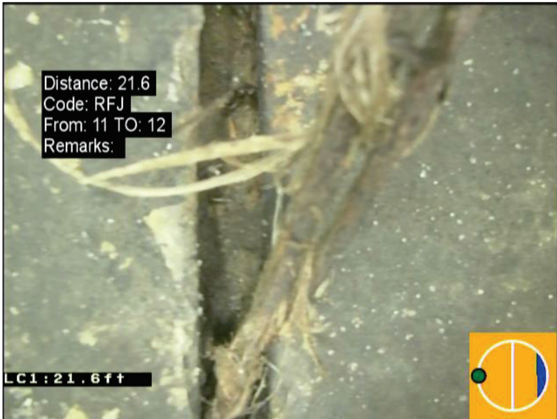
June 13, 2024 – Pacific Highway Crossing pipe separation due to tree roots
