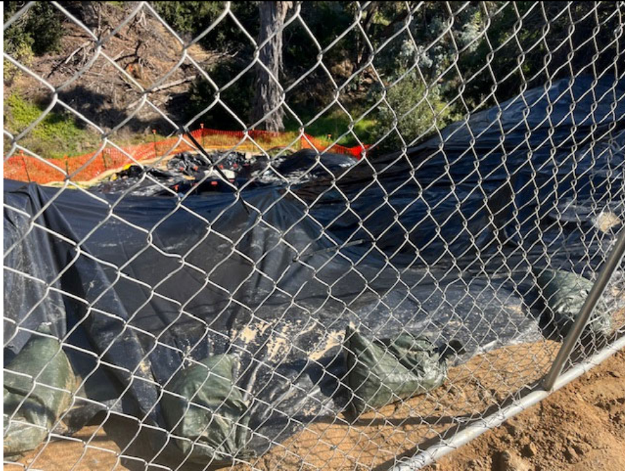
Photo 1. The impact area after the completion of work activities, taken from the residential backyard. View east.
