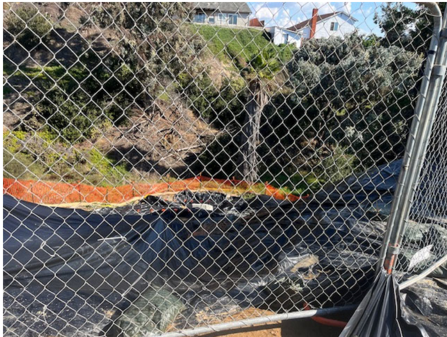
Photo 2. The impact area after the completion of work activities, taken from the residential backyard. View east.
