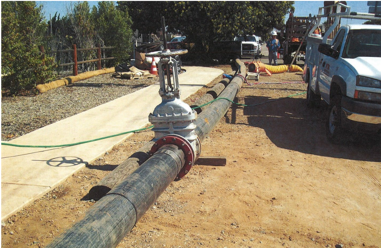
KTA Project – City of San Diego Otay Valley Sewer Manhole Rehabilitation (Phase 1 & 2)
