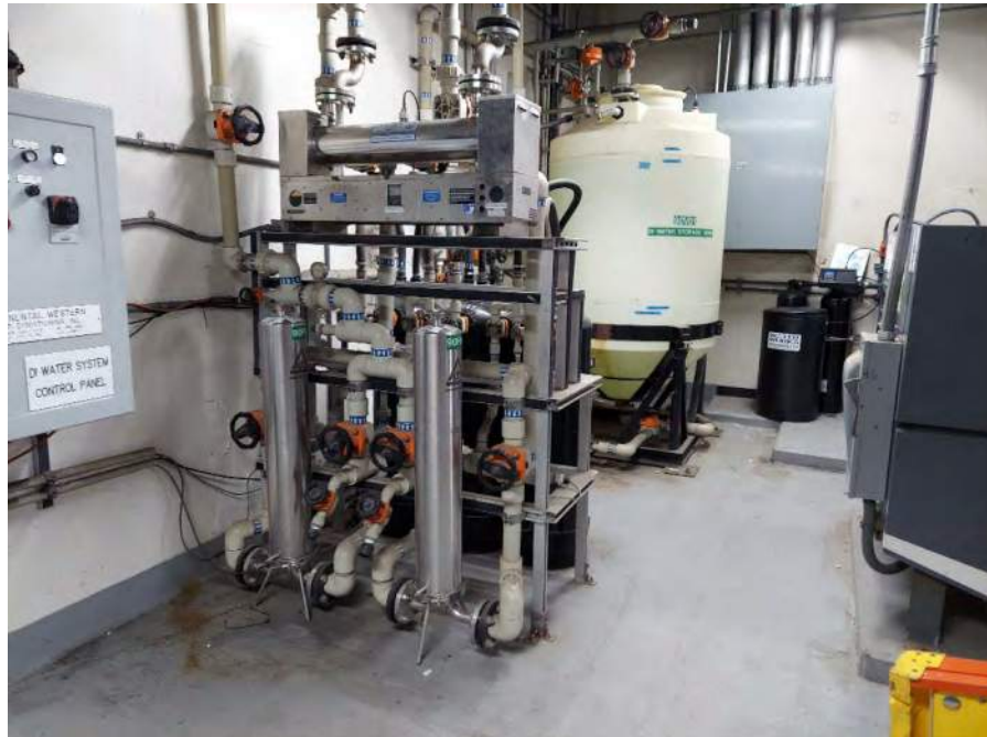
Photograph 25: View of deionized (DI) water system in the utility room on the first floor of the main building.
