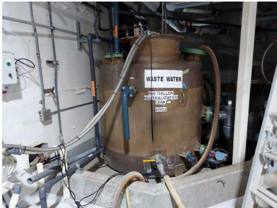
Photograph 28: View of the 500-gallon waste water neutralization tank in the utility room on the first floor.
