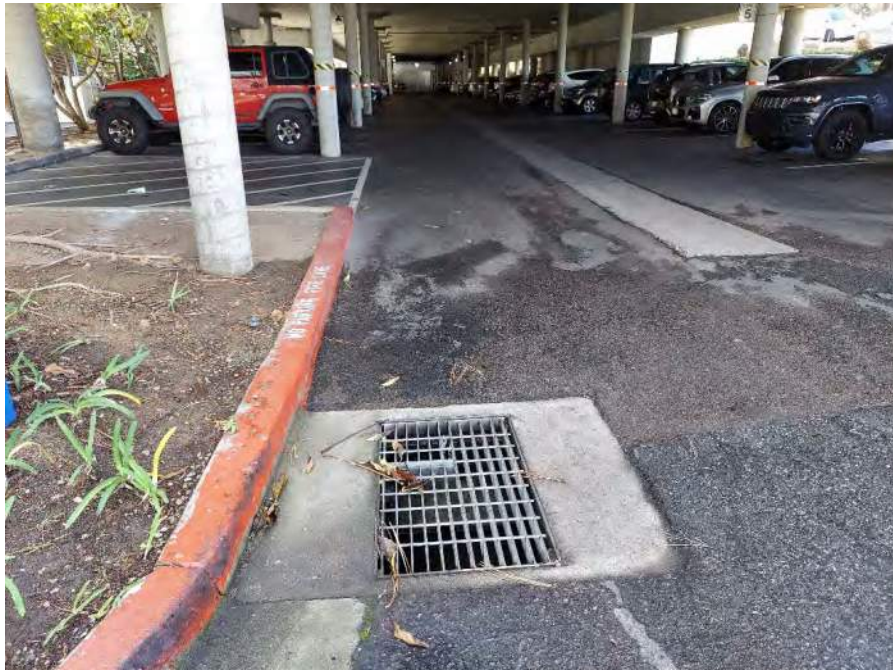
Photograph 31: View of a storm drain at the northwest portion of the site and the first level parking lot, facing south.
