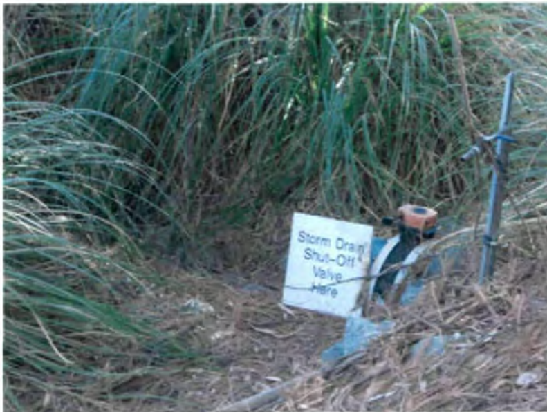
Photo 4: Storm drain emergency s hut-off valve located at the southeast end of the facility.
