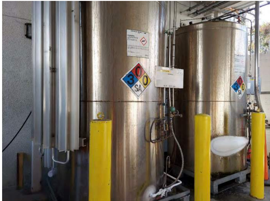
Photograph 27: View of refrigerated nitrogen tanks adjacent to the utility room on the first floor.
