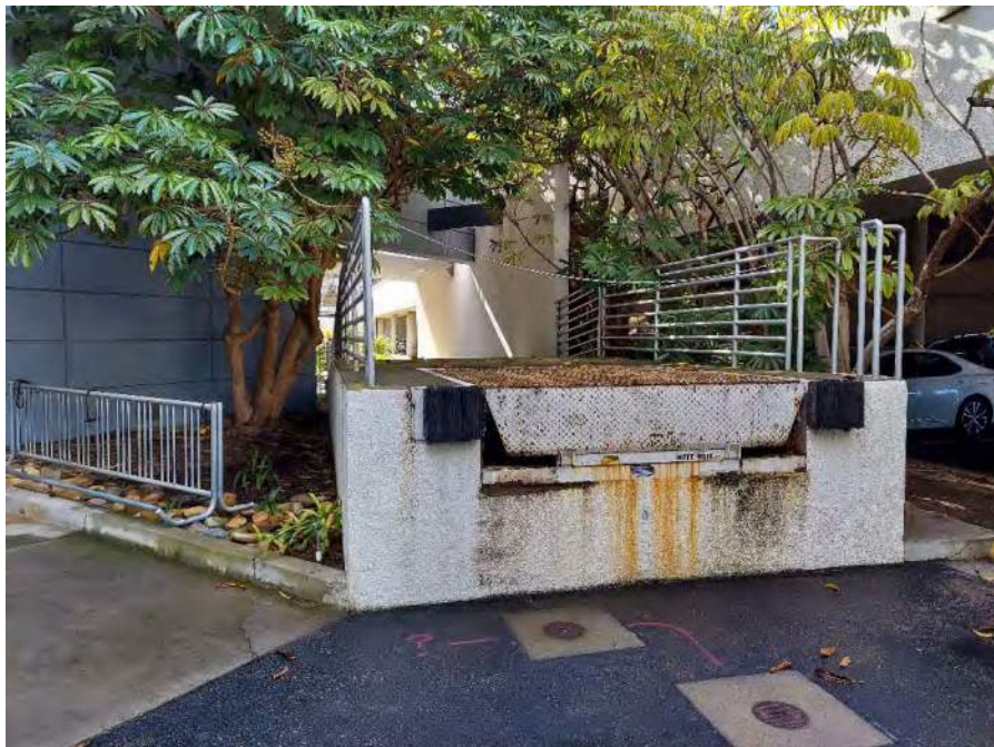
Photograph 30: View of the loading dock on the northwest portion of the site, facing south.
