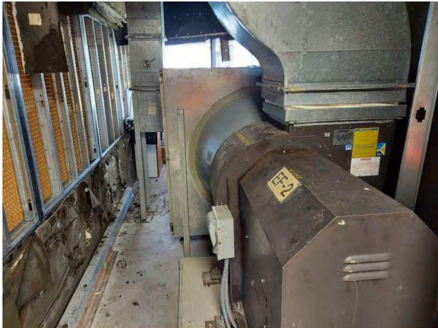
Photograph 5: View of an exhaust fan blower on the second floor.
