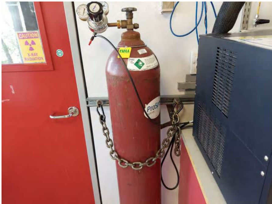
Photograph 14: View of 304 cubic-foot compressed nitrogen cylinder in a lab space on the first floor.
