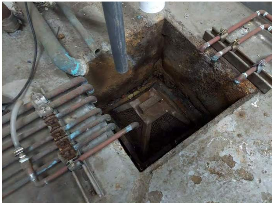
Photograph 26: View of condensate drain in the utility room on the first floor.
