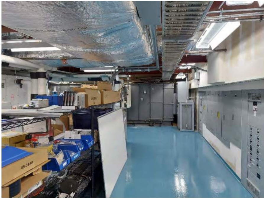
Photograph 9: View of maintenance equipment storage in the mezzanine on the second floor.
