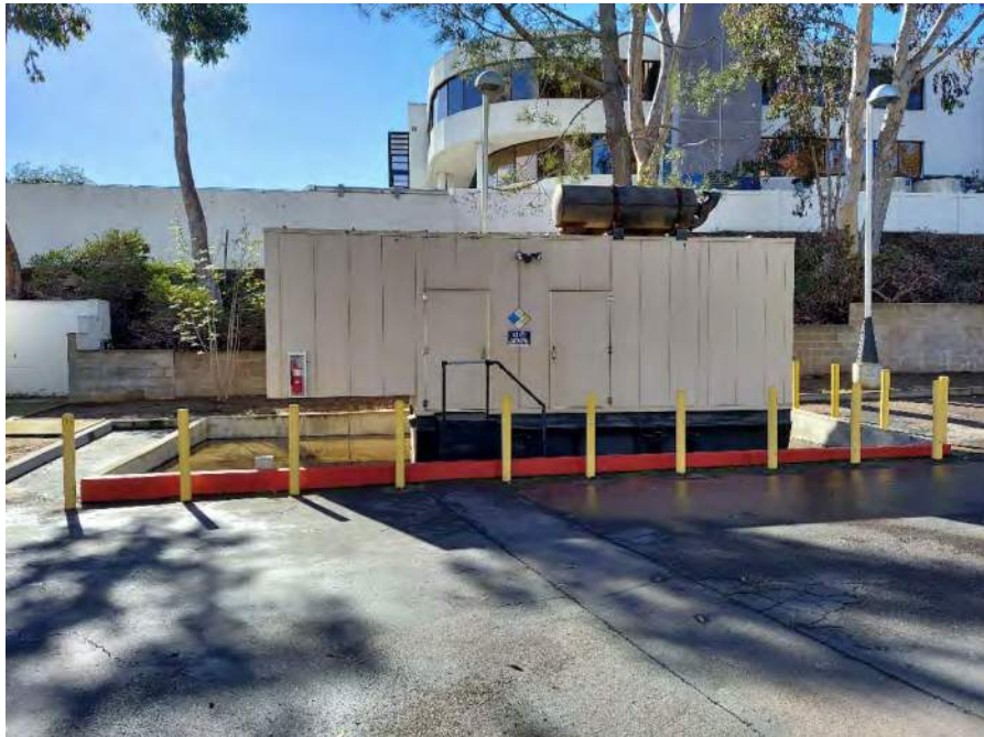
Photograph 24: View of the emergency generator at the southern end of the site, facing south.
