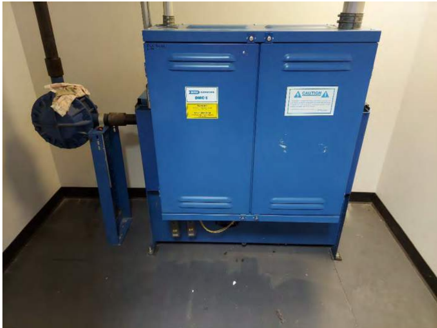
Photograph 29: View of the elevator equipment room on the first floor.
