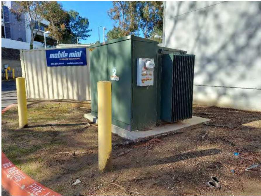
Photograph 23: View of a pad-mounted transformer at the rear of the main building, facing west.
