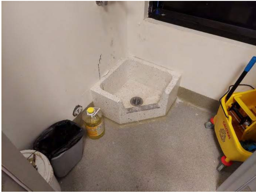
Photograph 11: View of the mop sink in a janitor's closet on the first floor.
