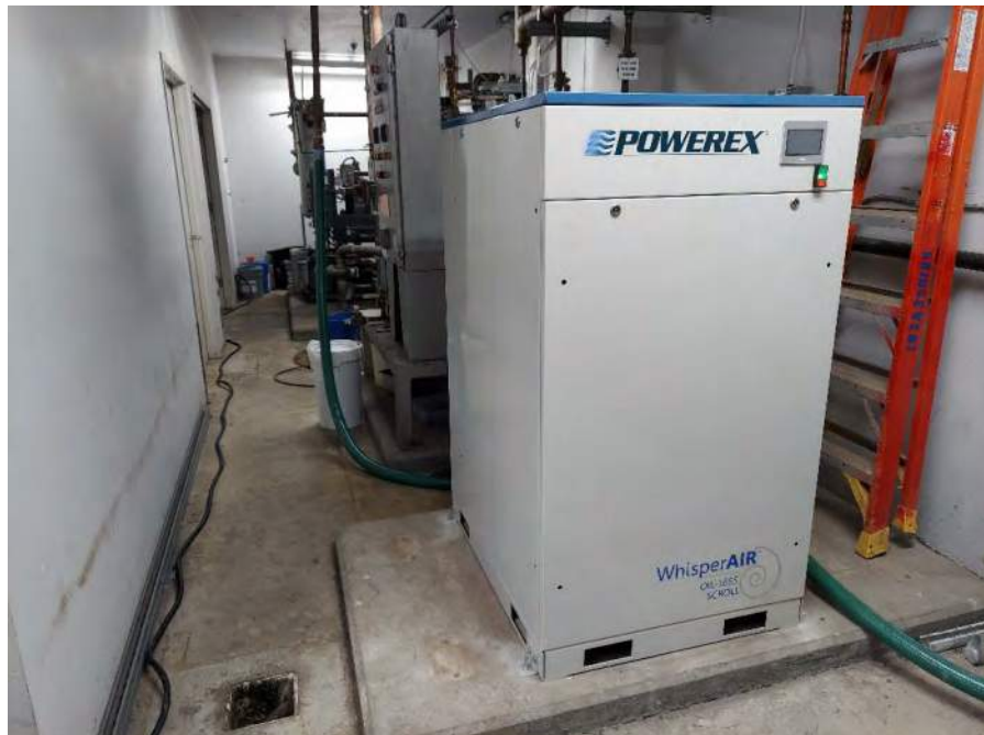
Photograph 16: View of an air compressor (right) and liquid ring vacuum pump system (left) in the basement below the main two-story building.
