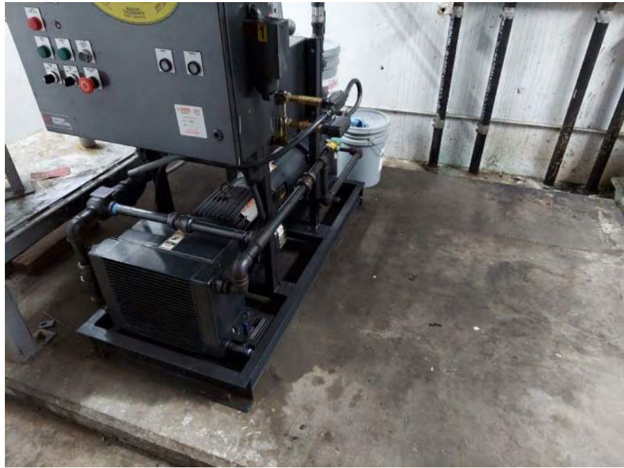
Photograph 17: View of stained concrete near the vacuum pump system in the basement.
