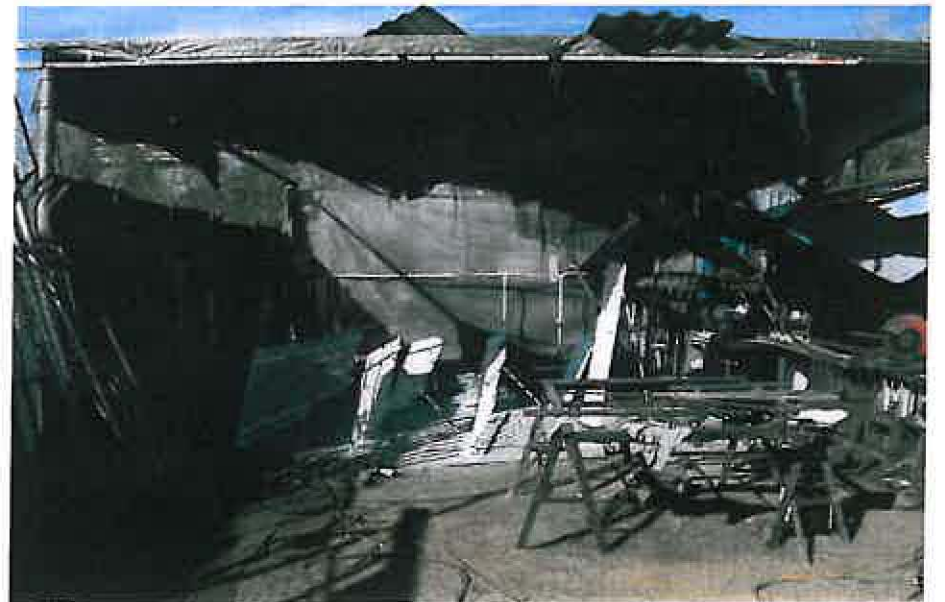
12. Paint spray area at Monroy's Towing on the western portion of the Property.
