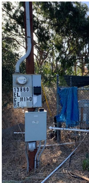
Photograph 14. Smaller electrical pole housing the meter box for the subject property.
