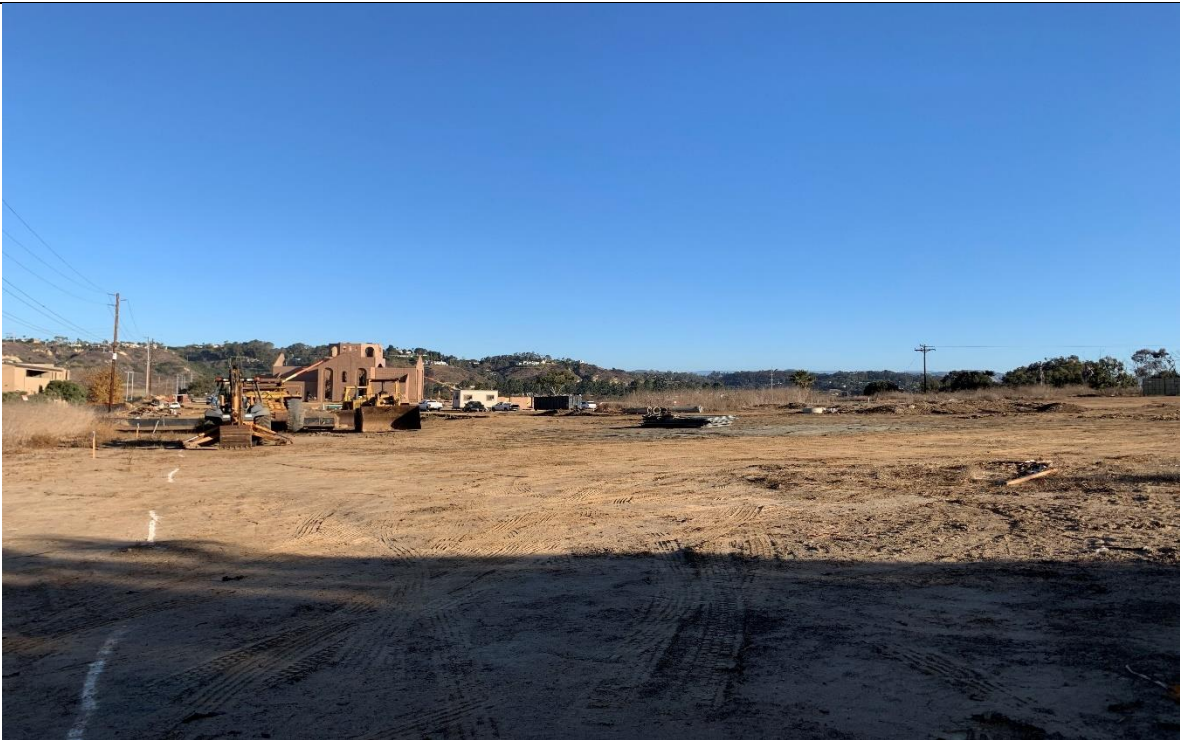
Photograph 1. Current construction project to the north of the subject property, provided site access.
