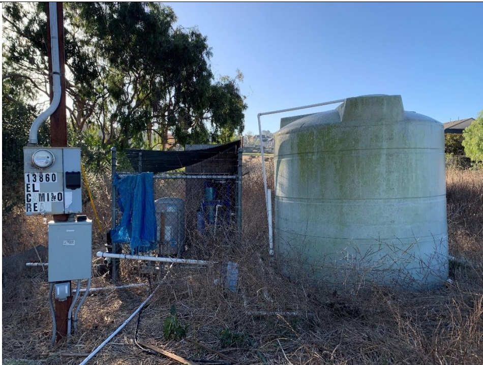
Photograph 7. Water storage tank in southeastern corner of the subject property.
