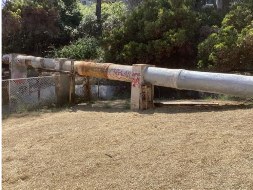
Photograph 9: Pacific Beach – Tourmaline Surf Park. Pipeline at bottom of undeveloped slope.
