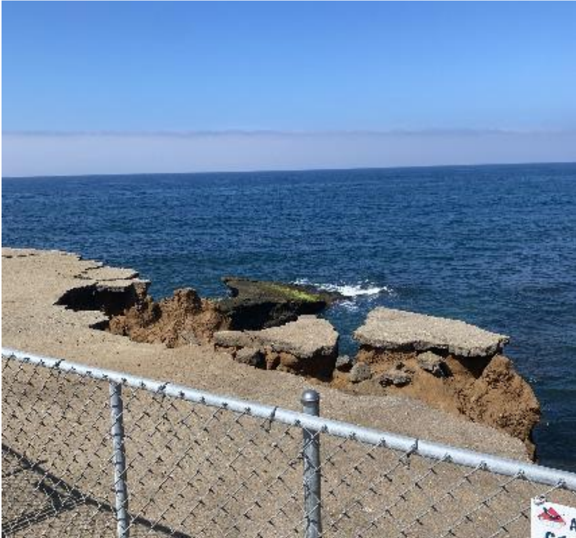
Figure 5.5-5. Eroding Cliffside on the Sunset Cliffs Project Site
