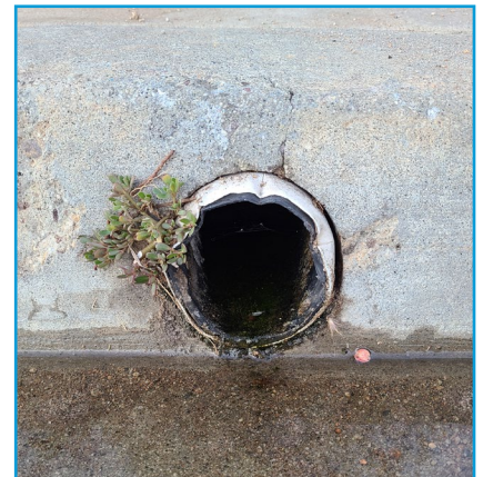
Warning signs of improper drainage.
