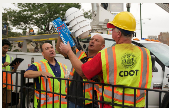
Installing AoT sensors, Chicago Source: University of Chicago, 2016
