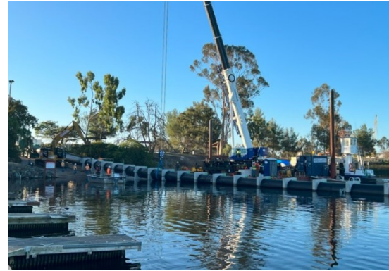
Pure Water construction crews are assembling the spine of the subaqueous pipeline.
