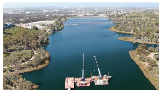
Barges remain on top of the Miramar Reservoir as construction continues below the surface.
