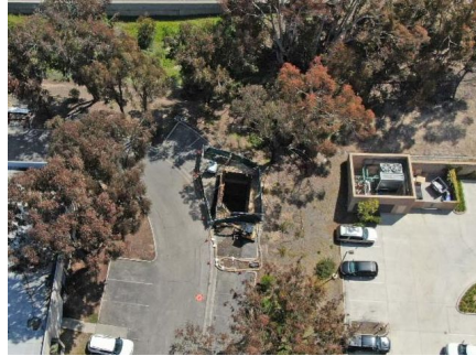
Construction continues on receiving shaft for the North City Pure Water Pipeline tunnel under Interstate 15.
