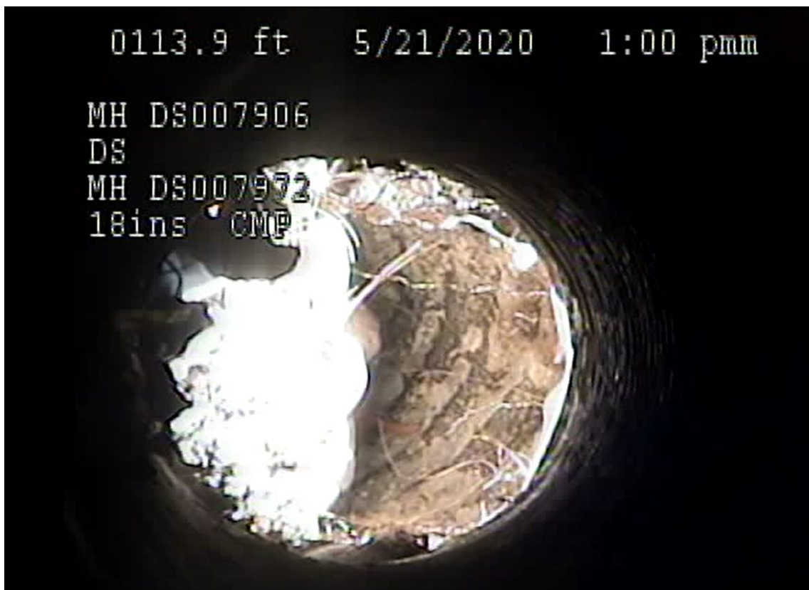
Collapsed CMPC at approximately 125-ft per CCTV from May 12, 2020
