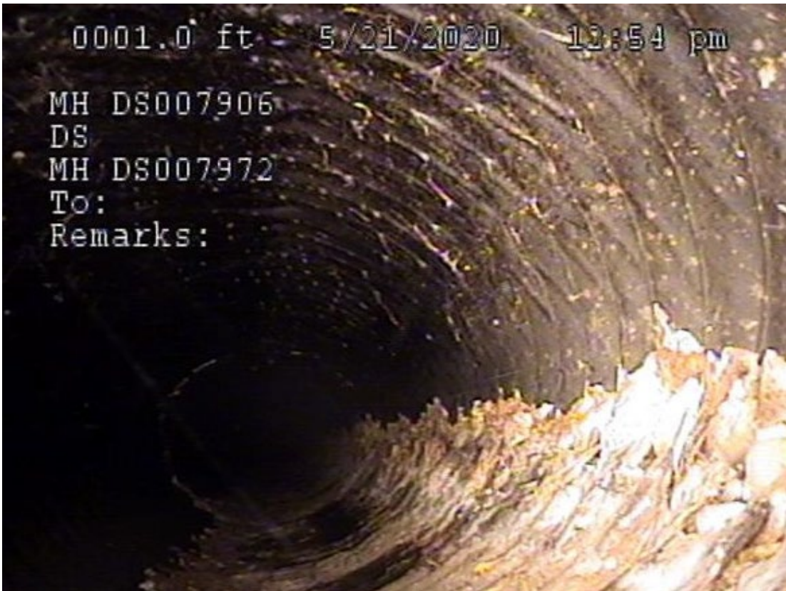
4 to 8 o'clock CMPC detachment per CCTV from May 12, 2020
