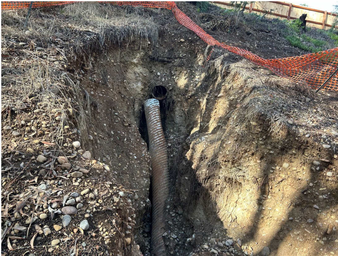
Upstream view of collapsed 18-in CMPC from hiking trail
