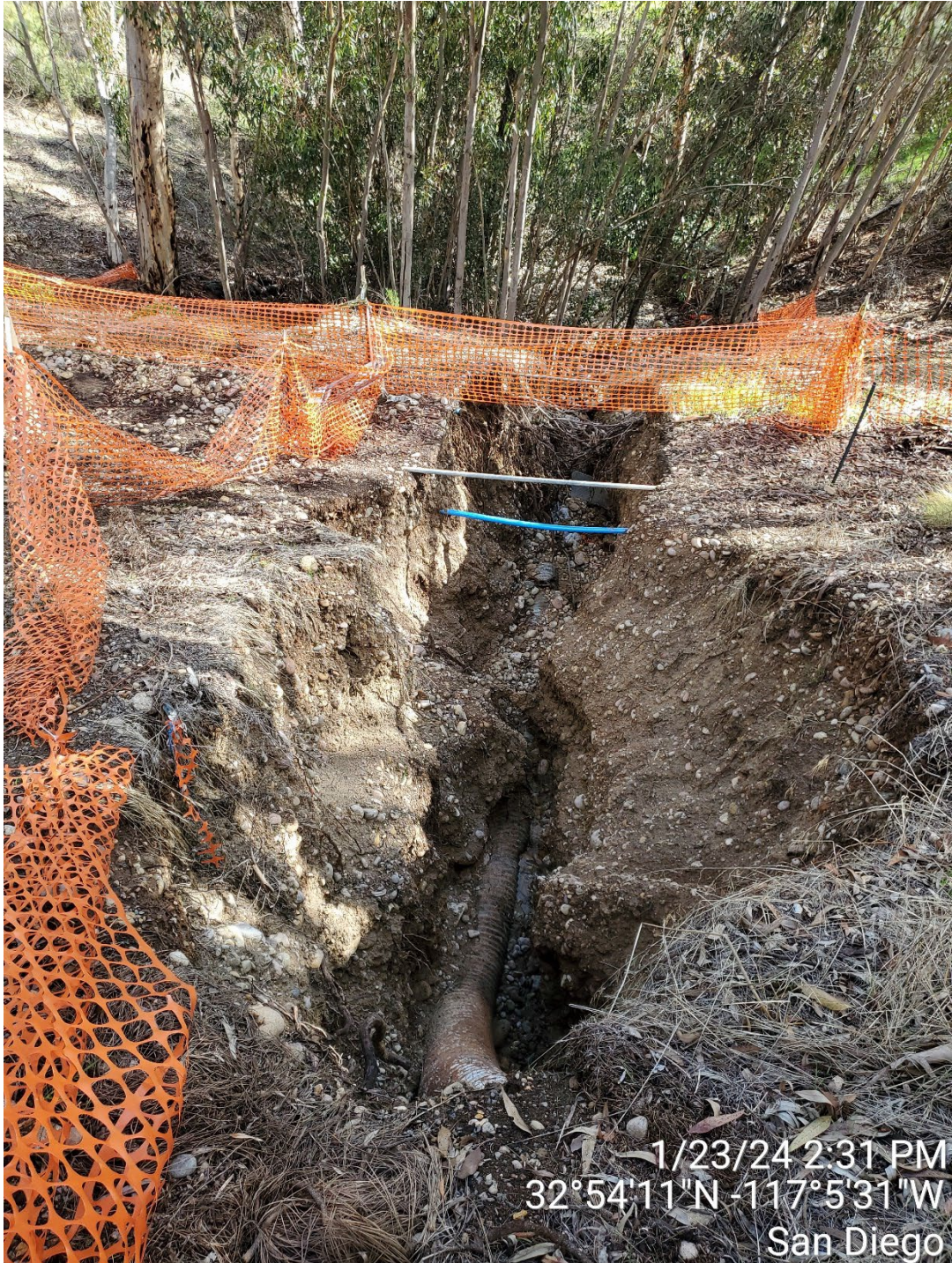
Downstream view of collapsed 18-in CMPC by property fences
