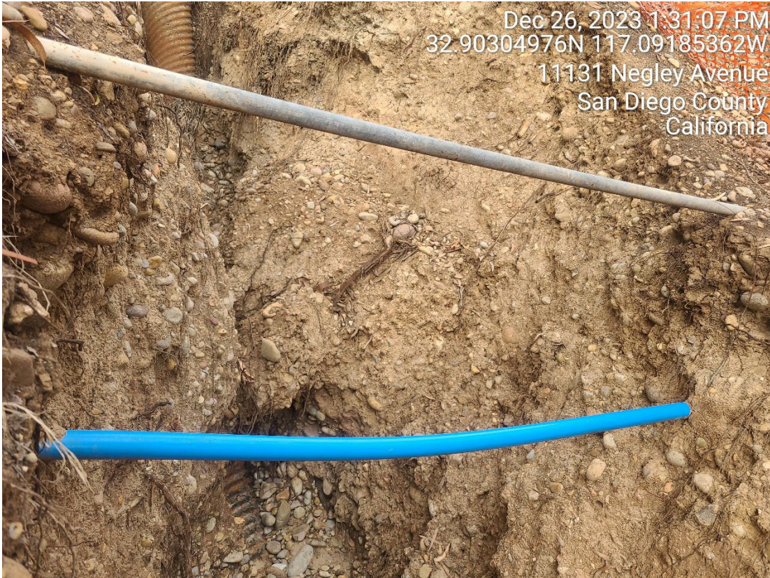
Undermined irrigation lines
