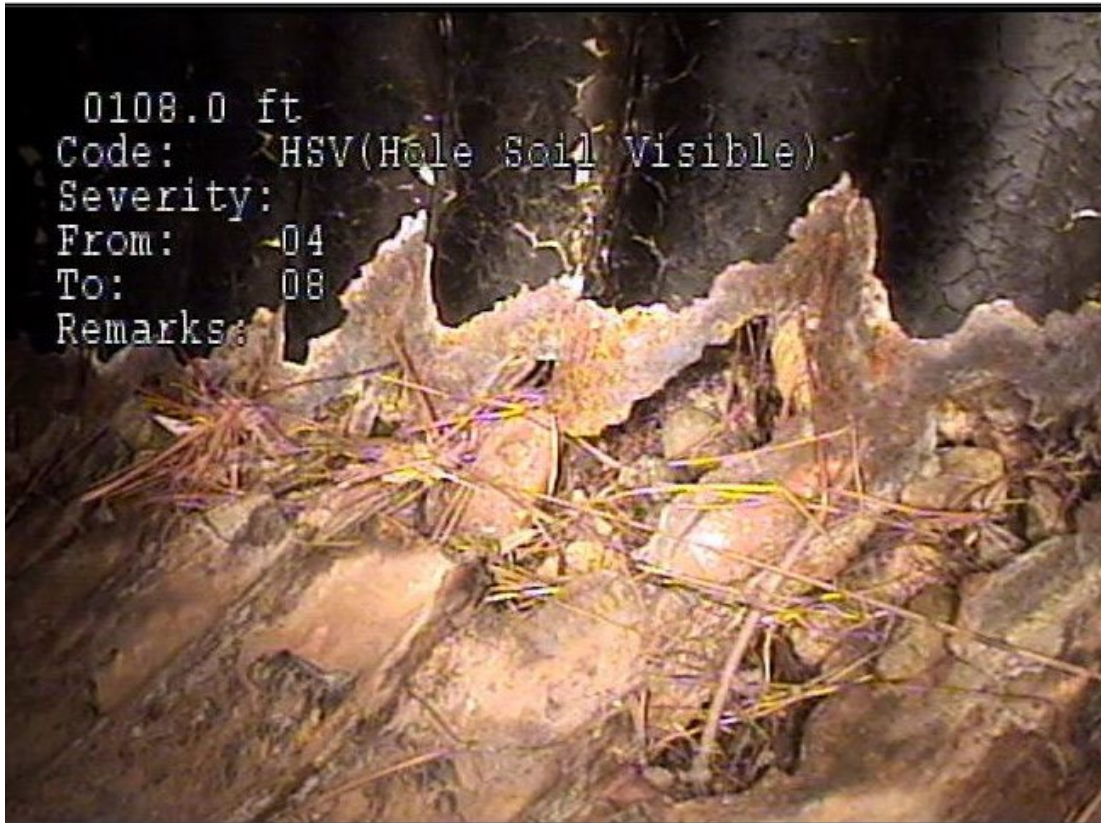
Detached pipe segments and soil visible per CCTV from May 12, 2020
