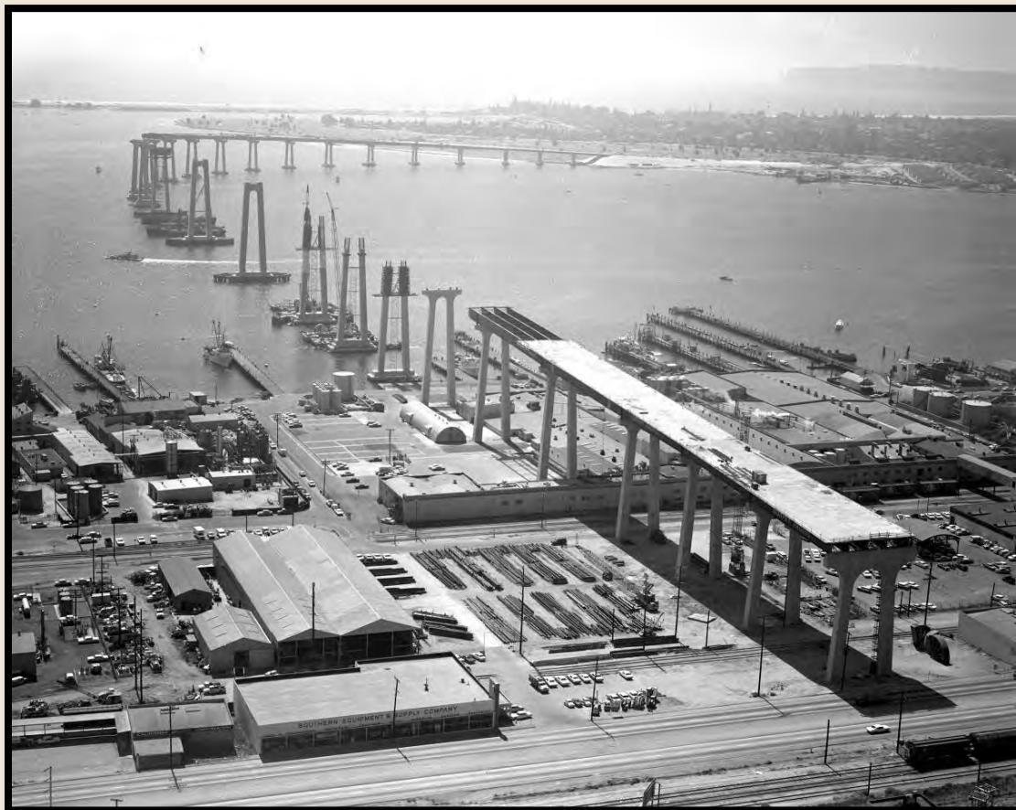
The Coronado Bridge Under Construction in 1968 (Courtesy of San Diego History Center)
