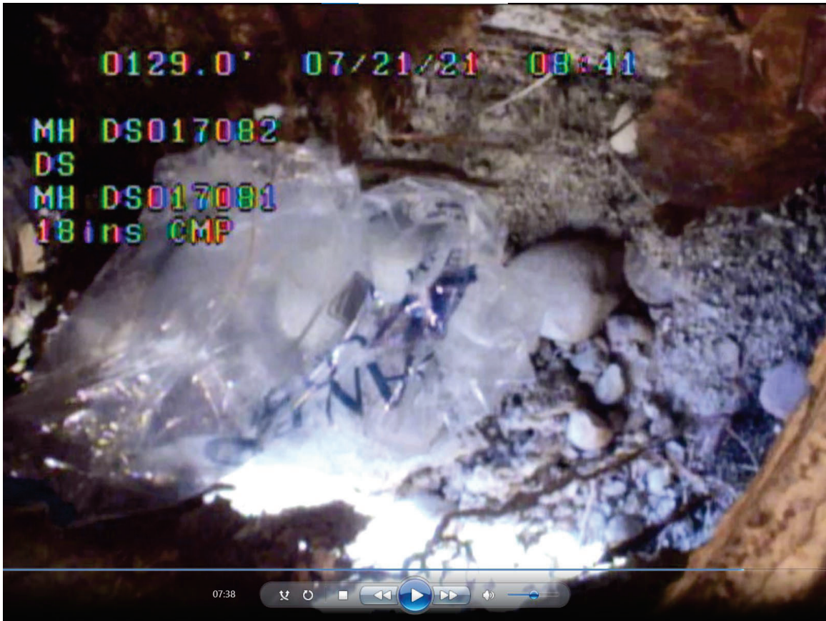
Void Visible from CCTV Survey on July 21, 2021
