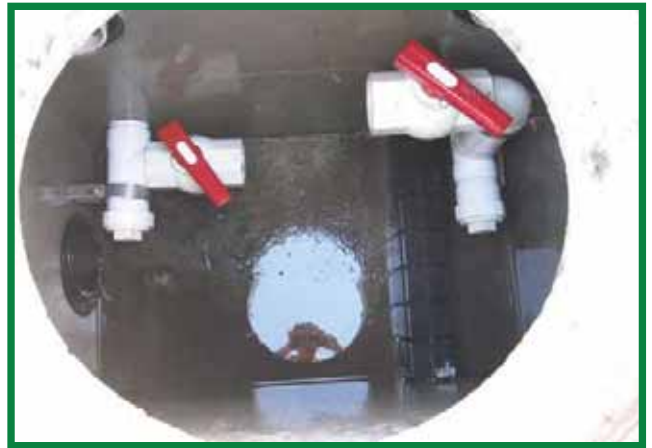
Open Discharge Chamber Lid to Assess Wetland Media Flow Rate and Replace Drain Down Filter Near Bottom
