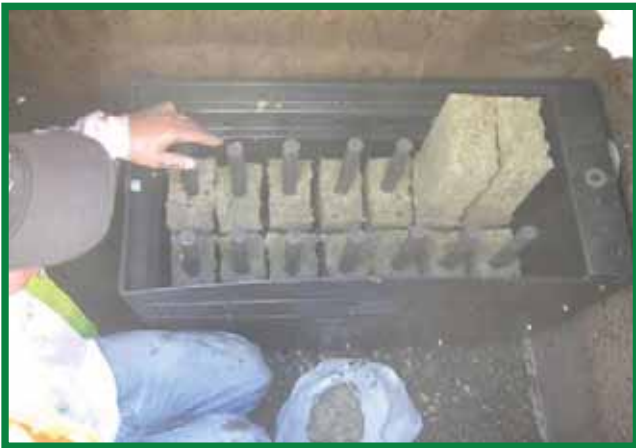
Replace with New BioMediaGREEN Filter Blocks and Replace Lid, then Catch Basin Filter and Replace Manhole or Grate
