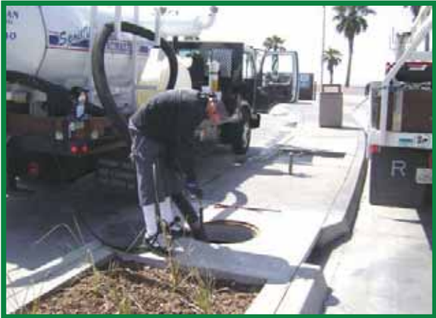
Access Pre-Treatment Chamber by Removing Manhole or Grate Cover
