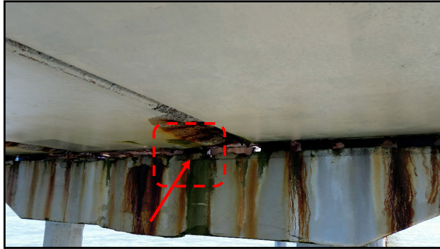
Photo 14: Bent 38 (looking east): Red arrow point to a displaced bearing at the middle plank that provides partial support.
