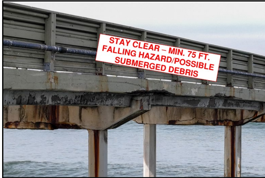
Figure 1: Proposed sign near missing Pile 45:B.
