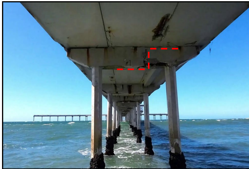
Photo 7: Bent 39 looking west. The red segmented line shows the vertical crack at the cold joint.
