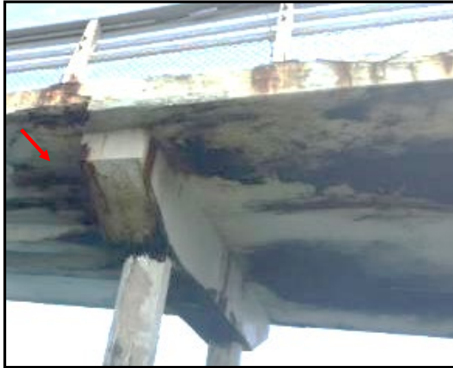
Photo 19: Bent 31 From July 2016 visual inspection looking north (underdeck spall partially hidden by pile cap).
