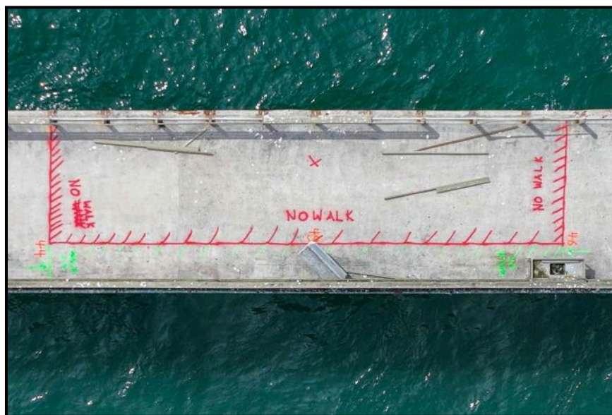
Photo 20: Walk/No walk demarcation around missing Pile 45:B
