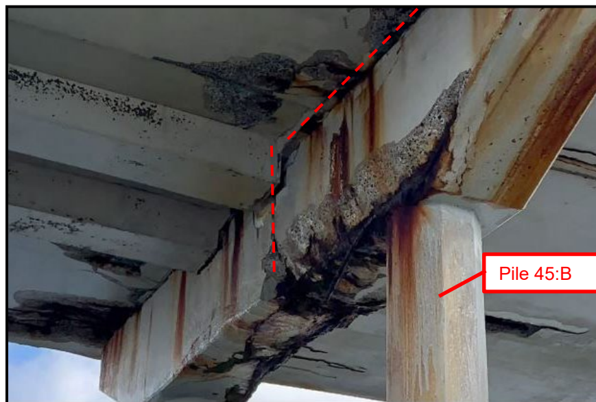
Photo 5: Bent 45 May 2023 visual inspection Dashed lines show assumed pile cap "break-away" location from pier deck.
