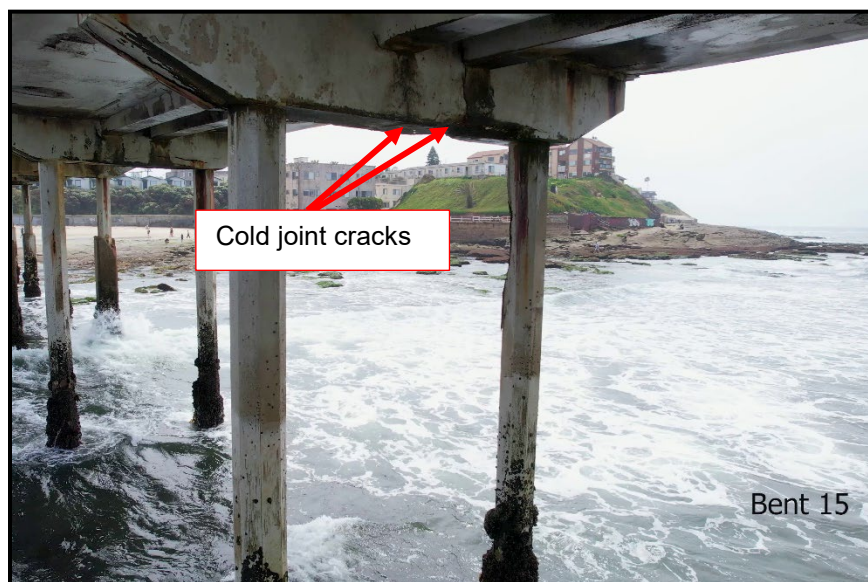
Photo 16: Bent 15 looking east. The red arrow points to initiation of cracking at cold joint.
