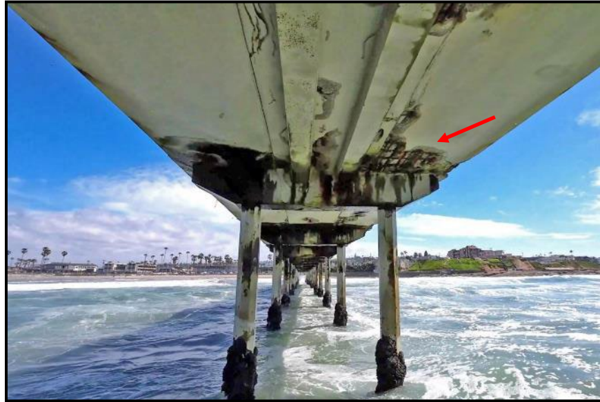
Photo 17: Bent 31 An elevation of pile cap at Bent 31 looking east (March 2024). The arrow points to the open spall corrosion with exposed strands at the southern plank.
