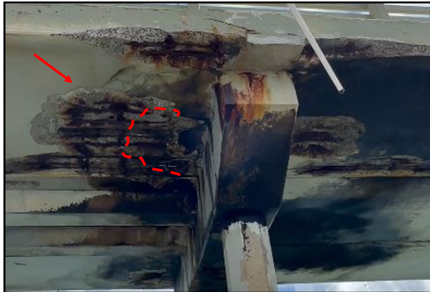
Photo 18: Bent 31 From May 2023 visual inspection looking north. The dashed line shows the approximate boundary of concrete damage when surveyed in 2016. The arrow points to the open spall corrosion with exposed strands at the southern plank during the 2023 survey.
