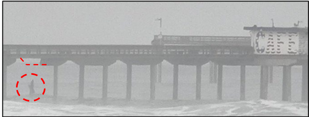
Photo 3: December 28th-29th, 2023 storm event. Pile 45:B broke (red circle) above the waterline pile cap broken shown in dashed red lines.
