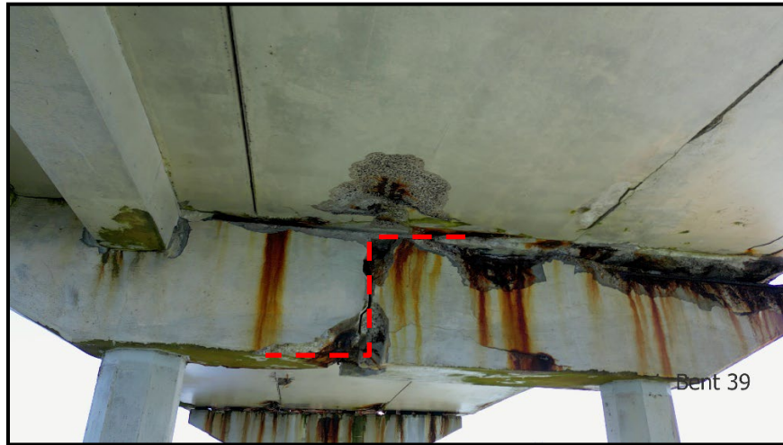
Photo 6: Bent 39 looking east. In the photo, spalled concrete is noticeable at the pile cap with exposed reinforcement at the top of the pile cap. The red segmented line shows the vertical crack at the cold joint.
