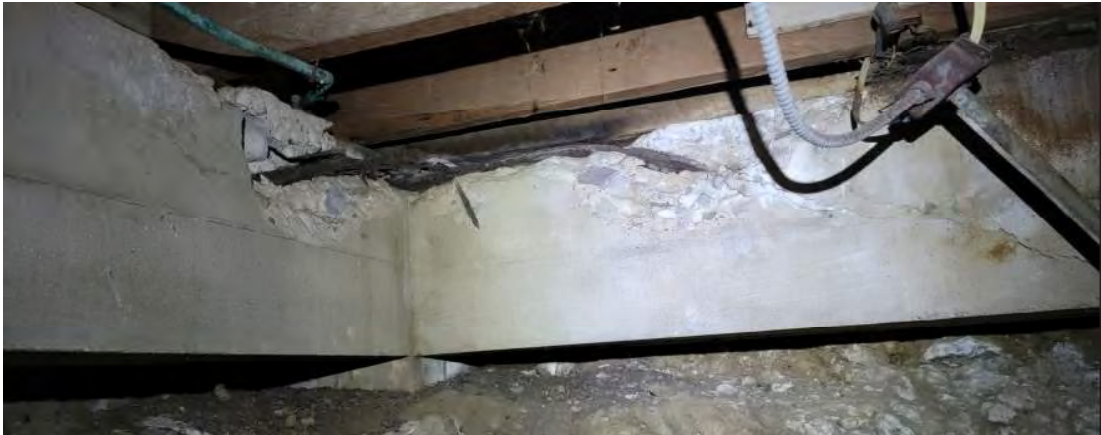
Figure 2 – Reinforcing shows substantial loss of area, Grade beams in South Wing
