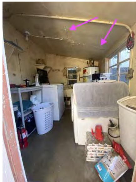
Figure B - Cracking in Garage Ceiling, Doors Racking
