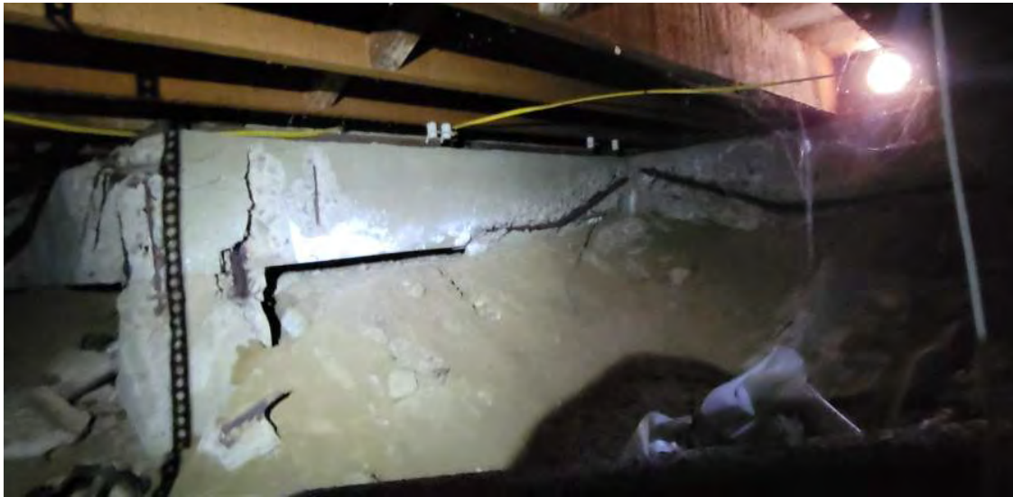
Figure 13 – Grade Beam and column showing significant deterioration. Reinforcement in corner has corroded and is completely broken.
