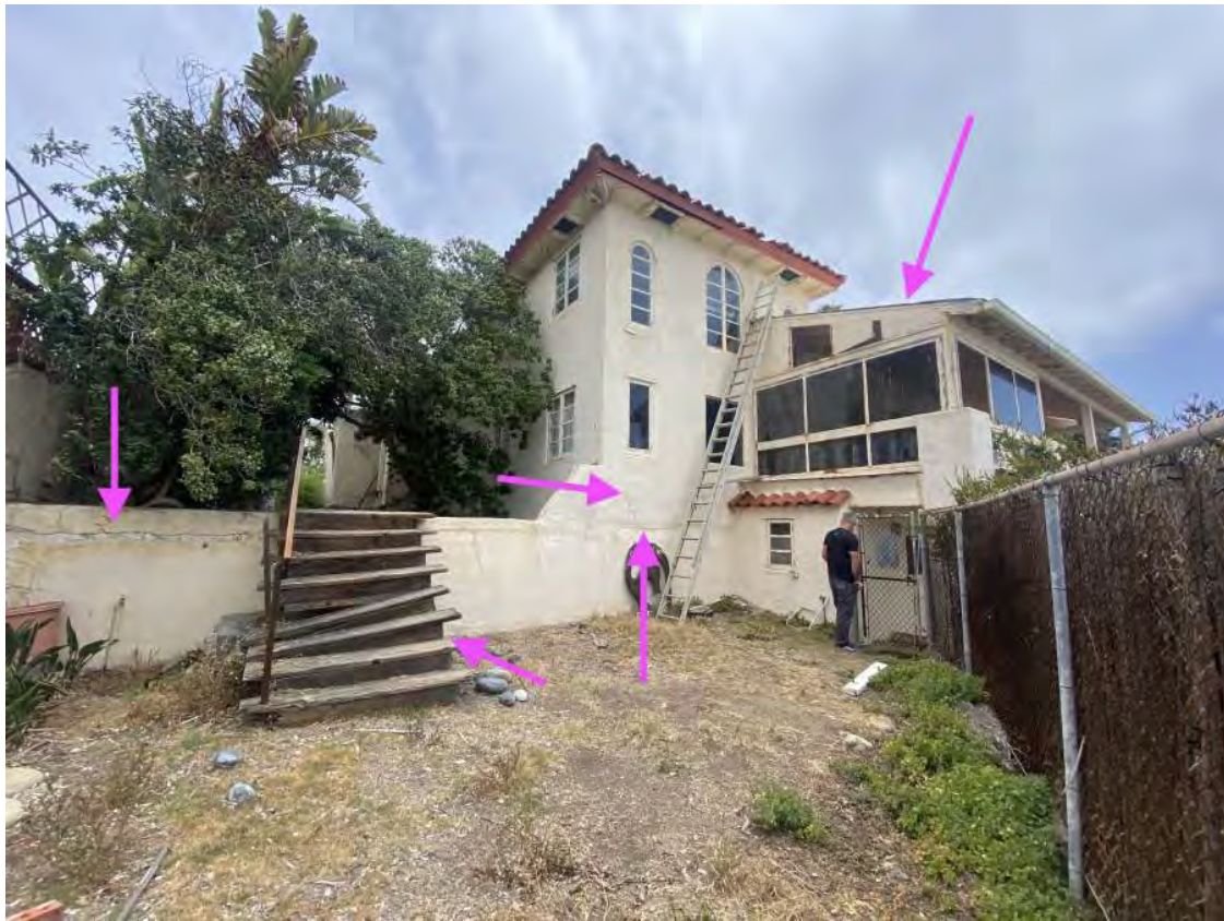
Figure A - Stairs Failing, Offset in Building Walls, Cracking in Multiple Site Walls
