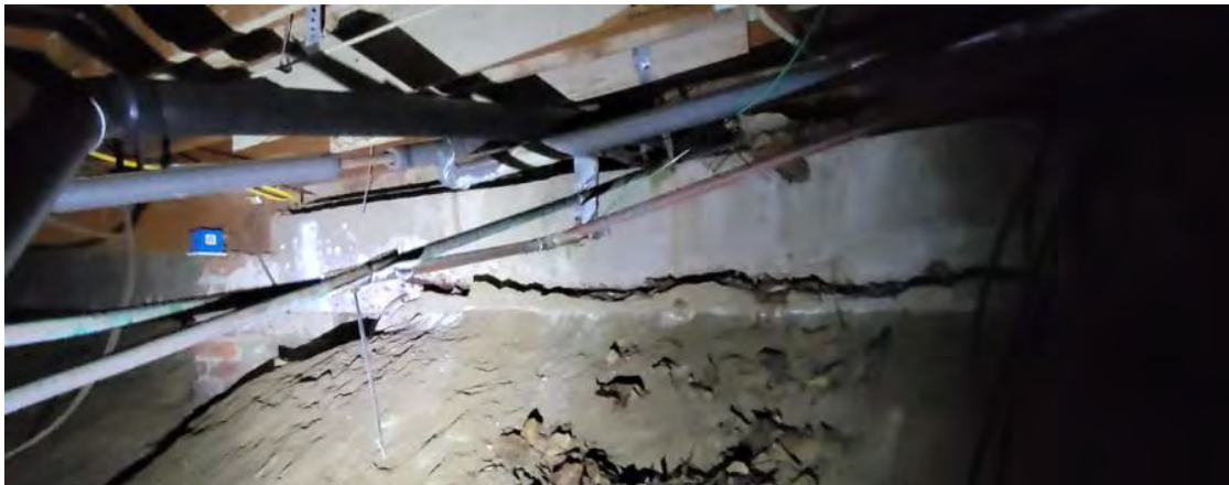
Figure 14 – Grade Beam showing significant spalling and corrosion. Reinforcement in bottom of beam is significantly corroded and exposed to soil. Beam is noticeable sagging.
