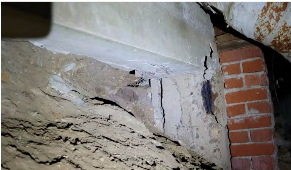
Figure 9 – Rebar Corrosion, Cracking and Spalling in Concrete Column and grade beam at North Wing. Note that both corners are spalling substantially as is blind side of beam.
