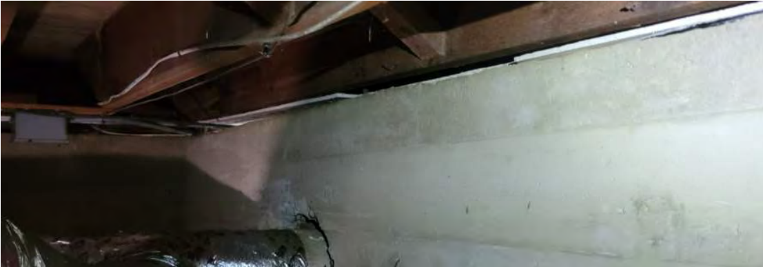
Figure 6 - West wall of South Wing, Wall on right slopes down towards the west with gap size increasing to the west. West portion of building appears to have settled and been shimmed to re-level structure above.
