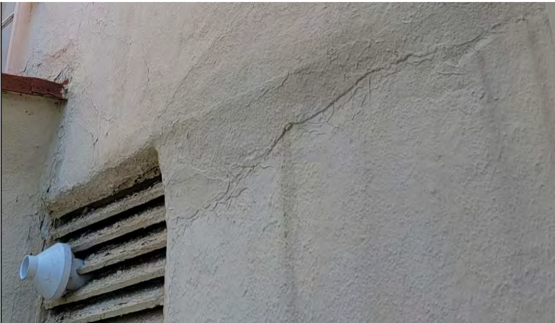
Figure 7 - Southwest Corner, Exterior, Appears to show patching of finish with movement of structure above relative to concrete walls/beams below.
