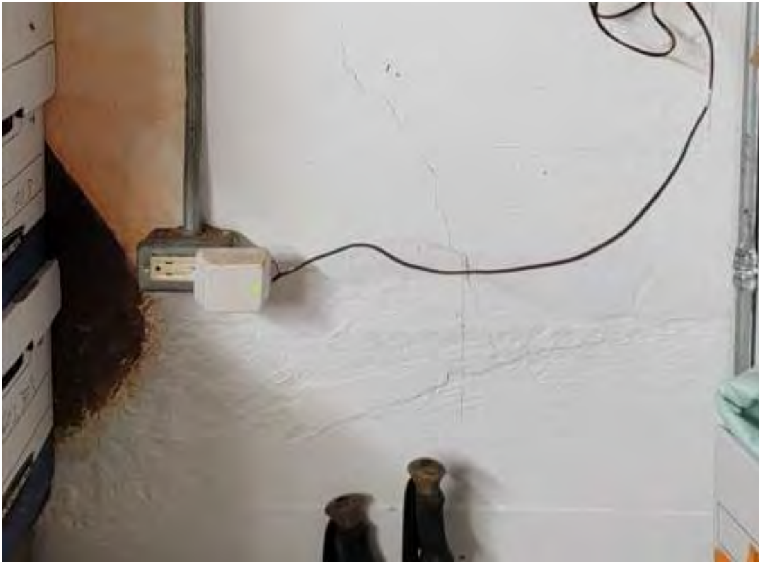
Figure 14 - Cracking of concrete basement walls in central lower level.
