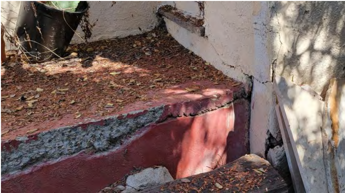
Figure 8 – Exterior Patio Area and Surrounding Walls Cracking and showing signs of settlement/distress.
