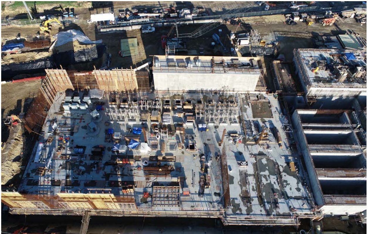
Pure Water project infrastructure (top and bottom).
