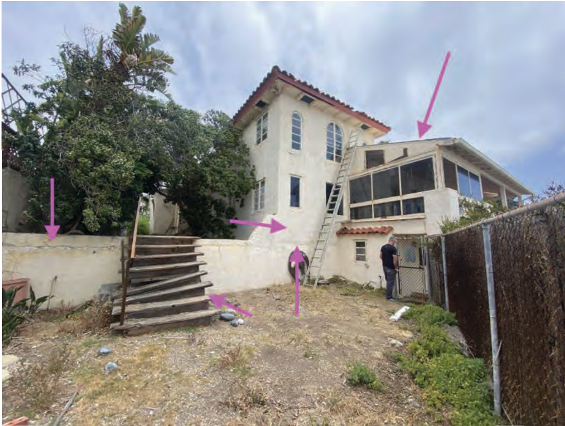
Figure A - Stairs Failing, Offset in Building Walls, Cracking in Multiple Site Walls
