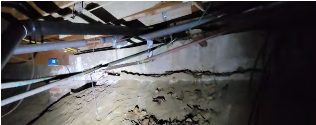
Figure 14 – Grade Beam showing significant spalling and corrosion. Reinforcement in bottom of beam is significantly corroded and exposed to soil. Beam is noticeable sagging.
