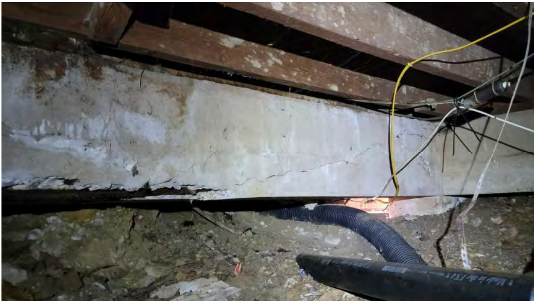
Figure 3 - Substantial Diagonal Crack (Shear), Spalling of Concrete, Corrosion of Rebar in South Wing Grade Beams.
