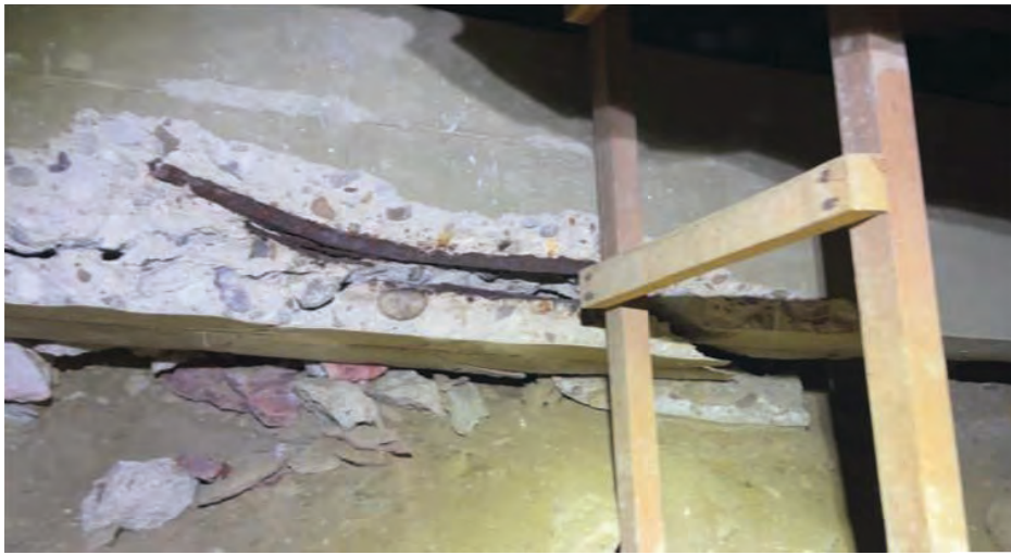
Figure B - Spalling, corrosion, delamination and displacement in a foundation beam.
