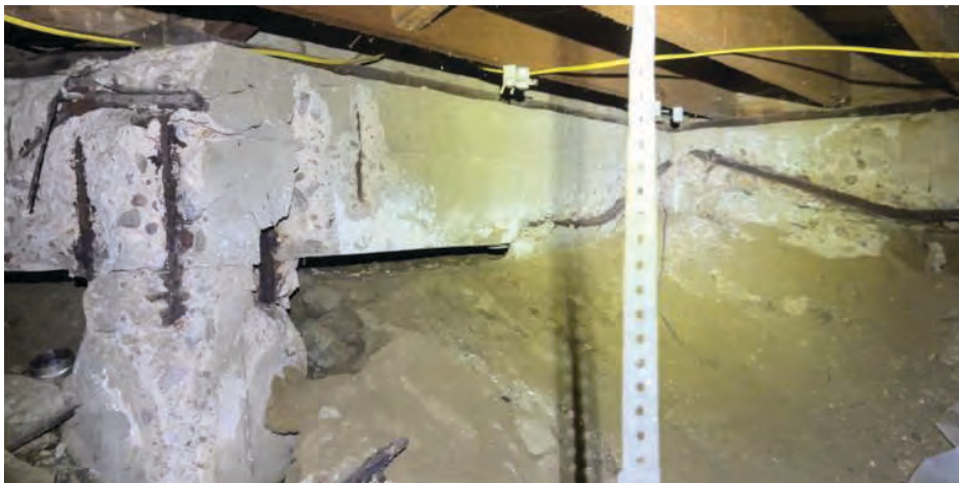
Figure A - Rebar Corrosion, Cracking and Spalling in Concrete Grade Beams at Western Portion of Building
