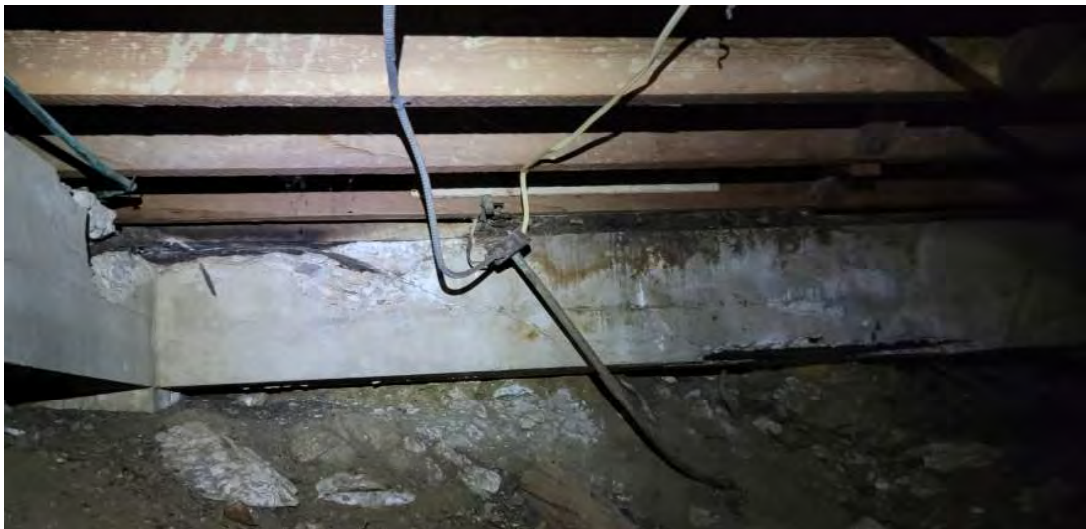
Figure 1 – Rebar Corrosion, Cracking and Spalling in Concrete Grade Beams at South Wing
