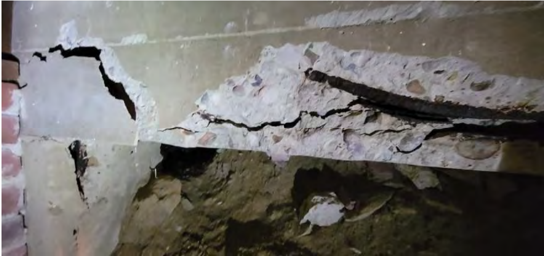
Figure 10 - Opposite End of Grade Beam shown in Figure 9 showing substantial spalling and corrosion
