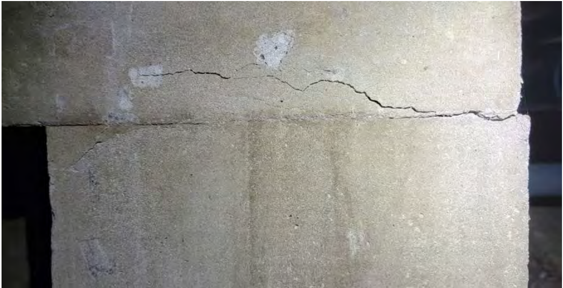
Figure 5 – Smaller Crack in Grade Beam/Column interface on Southwest Side
