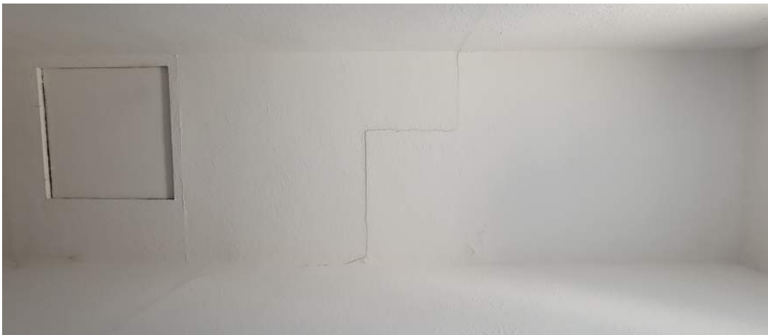
Figure 15 – Cracking of stair ceiling between main level and upper level. Cracking is indicative of building movement/settlement.
