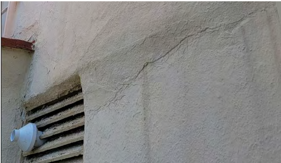
Figure 7 – Southwest Corner, Exterior, Appears to show patching of finish with movement of structure above relative to concrete walls/beams below.
