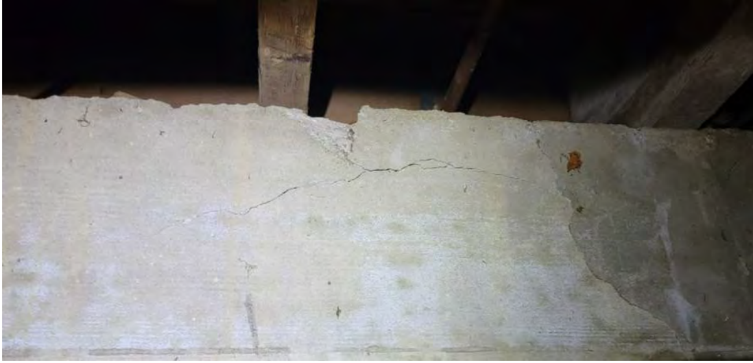
Figure 4 – Smaller Cracks in Grade Beam on Southwest side.
