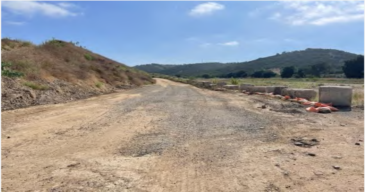
Facing east - walking underground transmission route. Adjacent to northern side of Beeler creek on dirt road. Northern pit will be dug in the dirt road.
