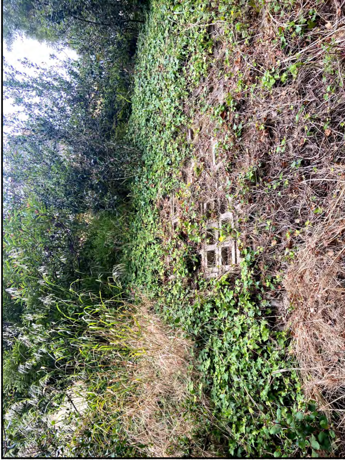
2. Concrete slope reinforcement on the Developed Land below the residence's lower terrace (from near southern boundary toward southeast).
