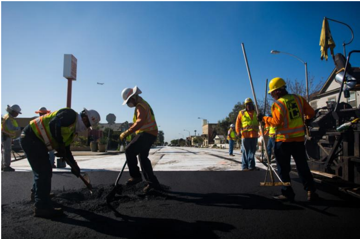
Construction crews working on utility undergrounding repave a street in South Park. / Photo by Dustin Michelson
