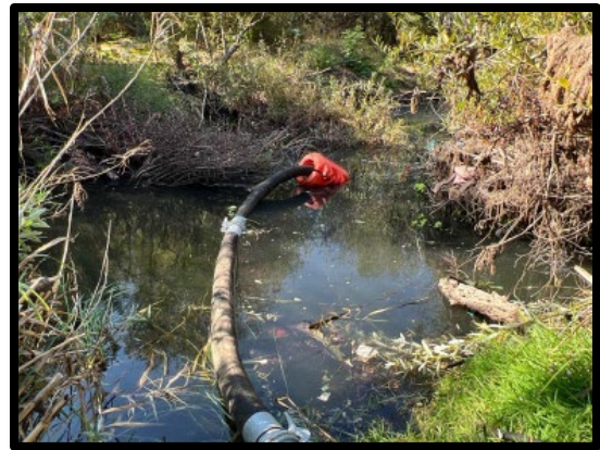
SR-163/6 th Ave Sewer Spill, September 2022
