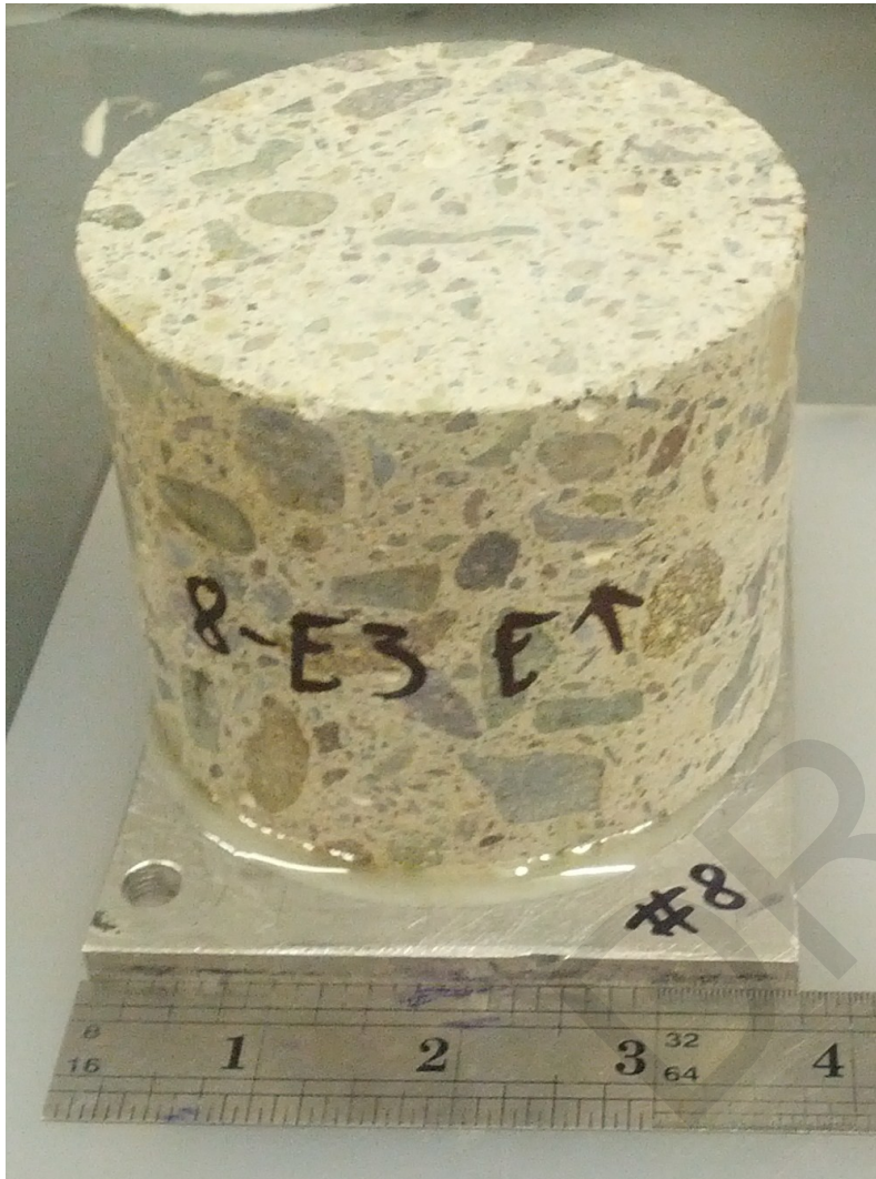
Core #8: Section for chloride analysis was cut at 2 1/2" from the exposure surface. No reinforcement was observed.
