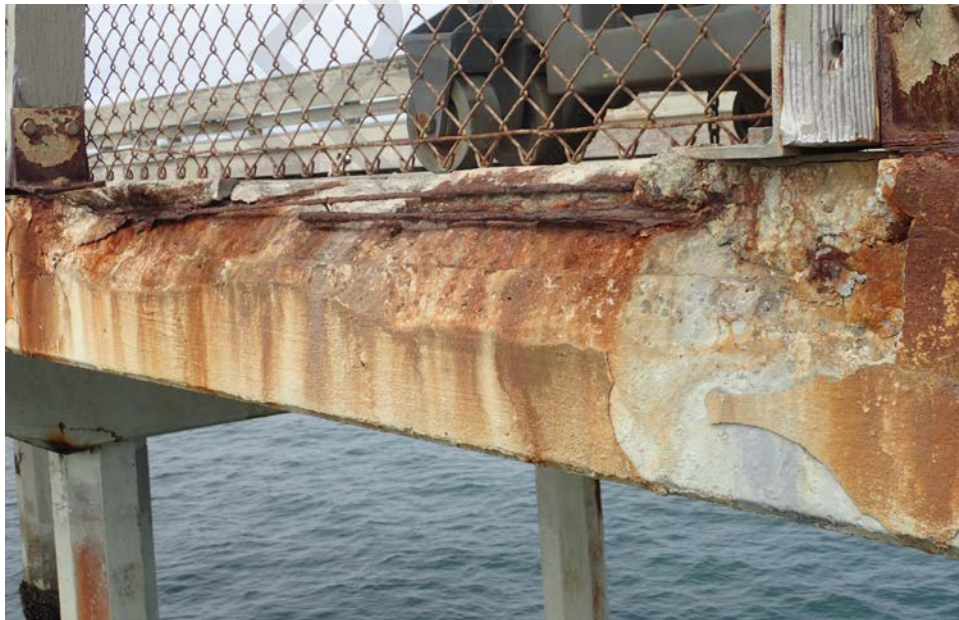
Figure 16 - Severe spalling of deck edge
