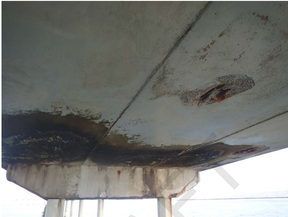
Figure 13 - Typical soffit damage
