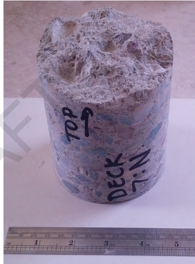
Core #1T: Section for chloride analysis was cut at 1 1/2" from the bottom surface. No reinforcement was observed.
