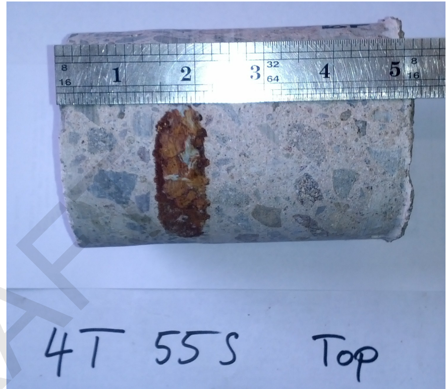
Core #4T: Section for chloride analysis was cut at the observed reinforcement level. Reinforcement is located at about 1 3/4" measured from the bottom surface (left hand side).
