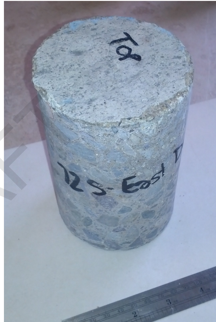
Core #5T: Section for chloride analysis was cut at 1 1/2" from the bottom surface. No reinforcement was observed.
