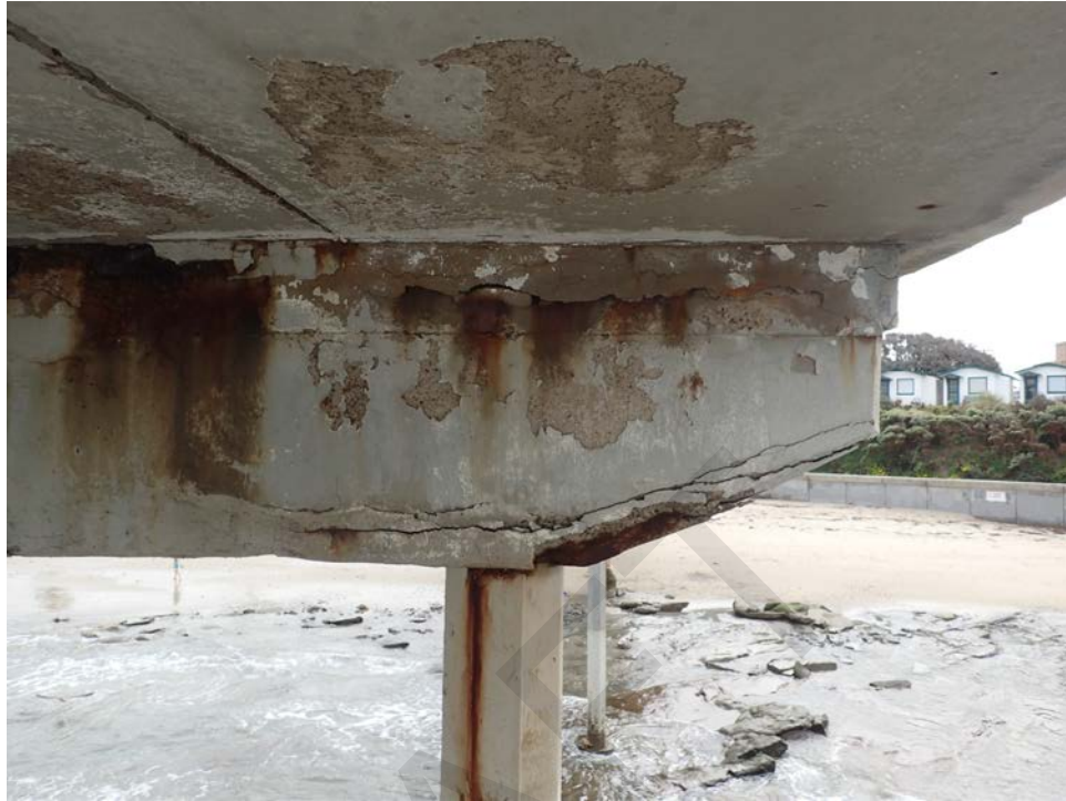
Figure 12 - Concrete spalling in the pile cap
