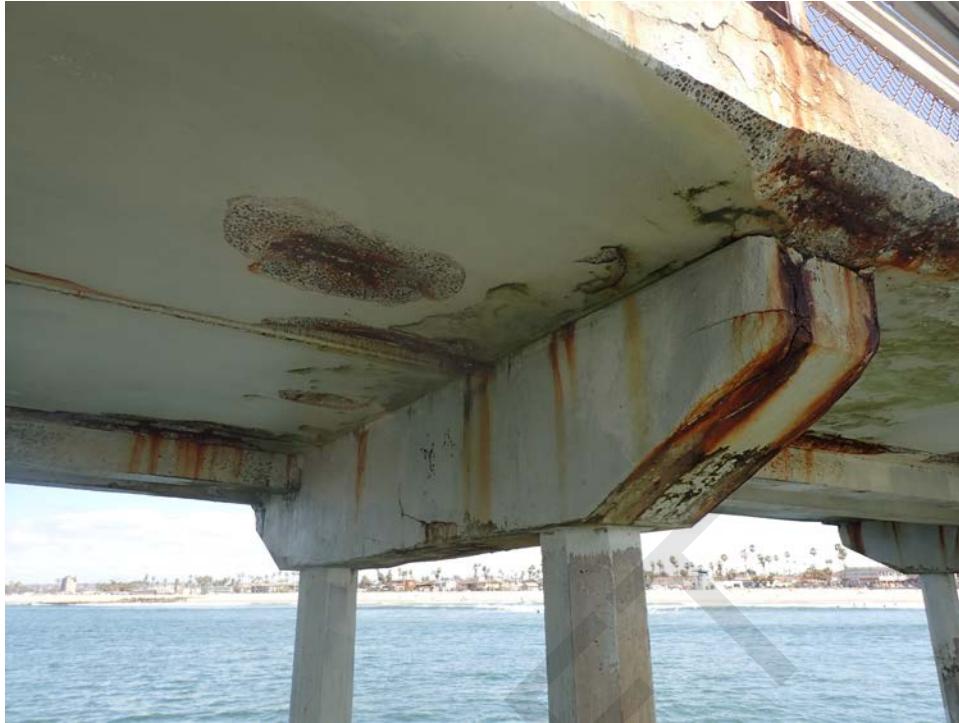
Figure 10 - Typical damage on pile cap
