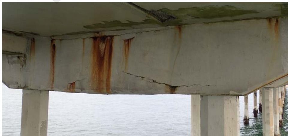
Figure 11 - Damage in cast-in-place portion of the cap
