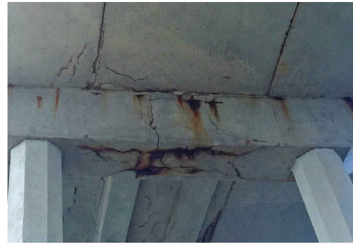
PILE CAP DAMAGE
