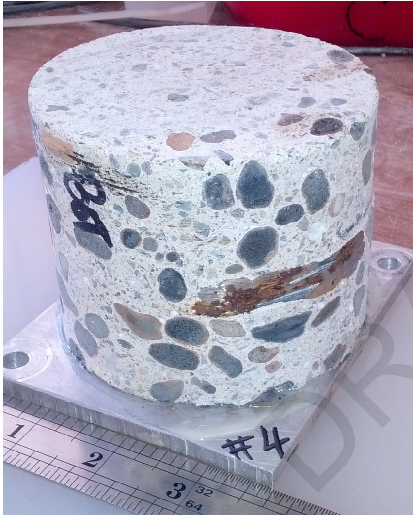
Core #4: Section for chloride analysis was cut at the observed reinforcement level. Reinforcement is located at about 1 5/8" below the exposure surface (bottom)
