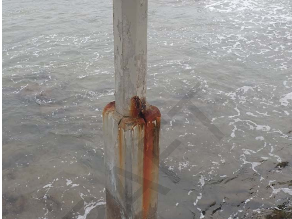
Figure 9 - Spalling at jacket (Pile 6N)
