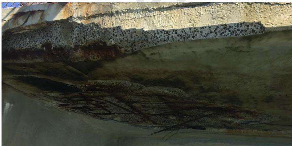
Figure 14 - Soffit at Bent 32 (Most extreme corrosion)
