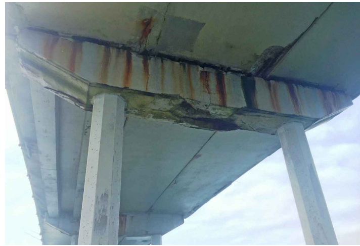
PILE CAP DAMAGE
