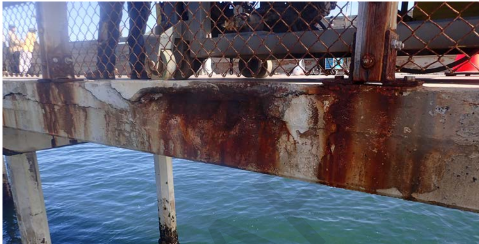
Figure 15 - Typical cracking in deck edge
