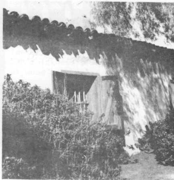
Typical double-hung wood window with wood head, jamb, and sill in plastered adobe wall. Note deep reveal of window, wood shutters, and plain chimney showing above the tile roof and pole rafters.
