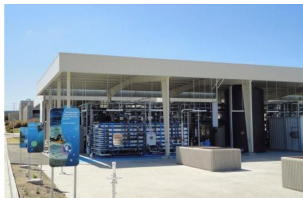
The advanced water purification facility is a component of the Water Purification Demonstration Project.
