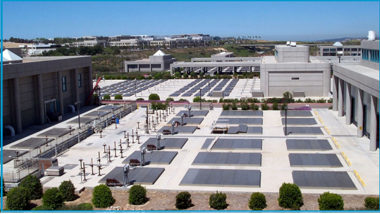
North City Water Reclamation Plant
