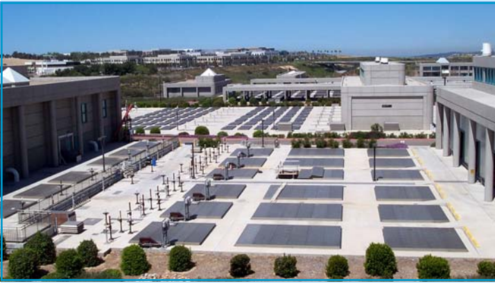
North City Water Reclamation Plant
