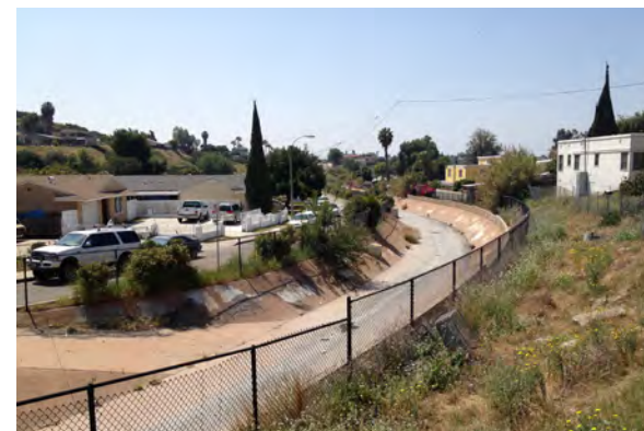
The primary natural feature within the study area, Chollas Creek, is channelized in many areas.
