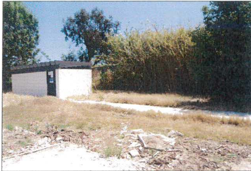
Verizon Tree/Equipment Area
