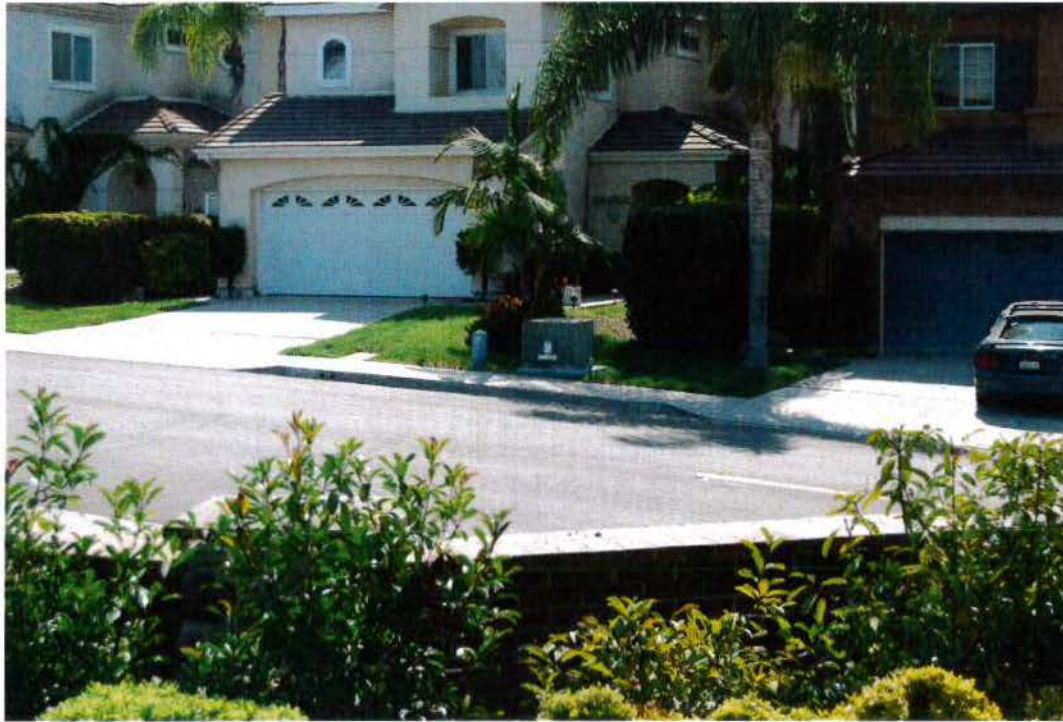
Proposed Utility Transformer
