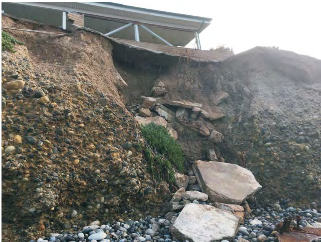
PHOTO 6A: Bluff below residence on February 4, 2021.
