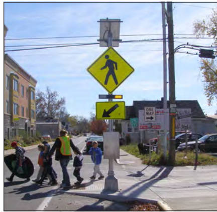
Rectangular Rapid Flashing Beacon
