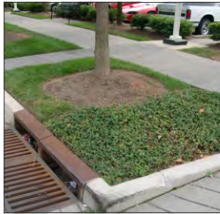
Tree Basin with Filters and Subsurface Drain
