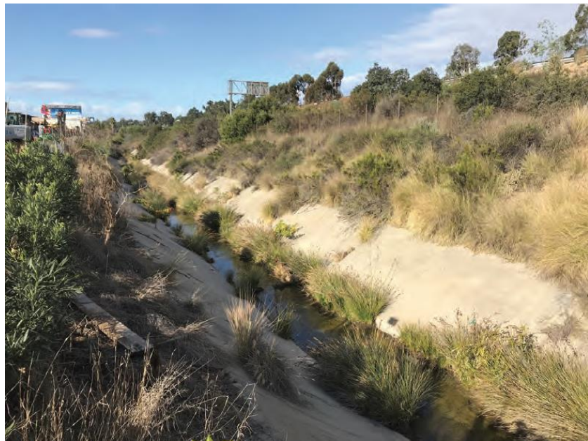
Photo 8. South Chollas Map 101 Channel Maintenance Project, pre maintenance, looking downstream (west) from east end of maintenance area, 2/21/2018.
