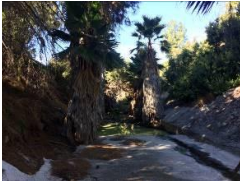
Photo 6. Montezuma Creek Channel Maintenance Project, pre- maintenance, facing west (downstream) toward fan palm stand and ponded surface water at the end of the concrete-lined channel, 04/24/2018
