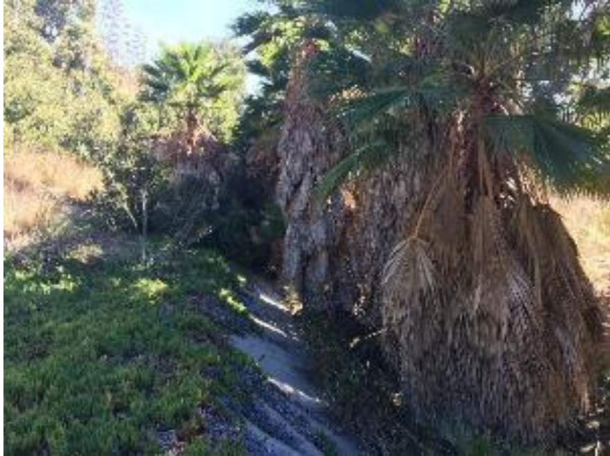
Photo 5. Montezuma Creek Channel Maintenance Project, pre- maintenance, facing east (upstream) toward Montezuma Creek Channel, 04/24/2018
