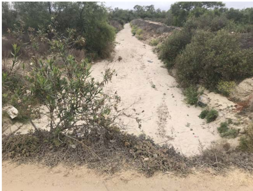
Photo 2. Tijuana River Valley Channel Maintenance Project, looking north into Smuggler's Gulch from the Disney Bridge, post maintenance, 05/11/18
